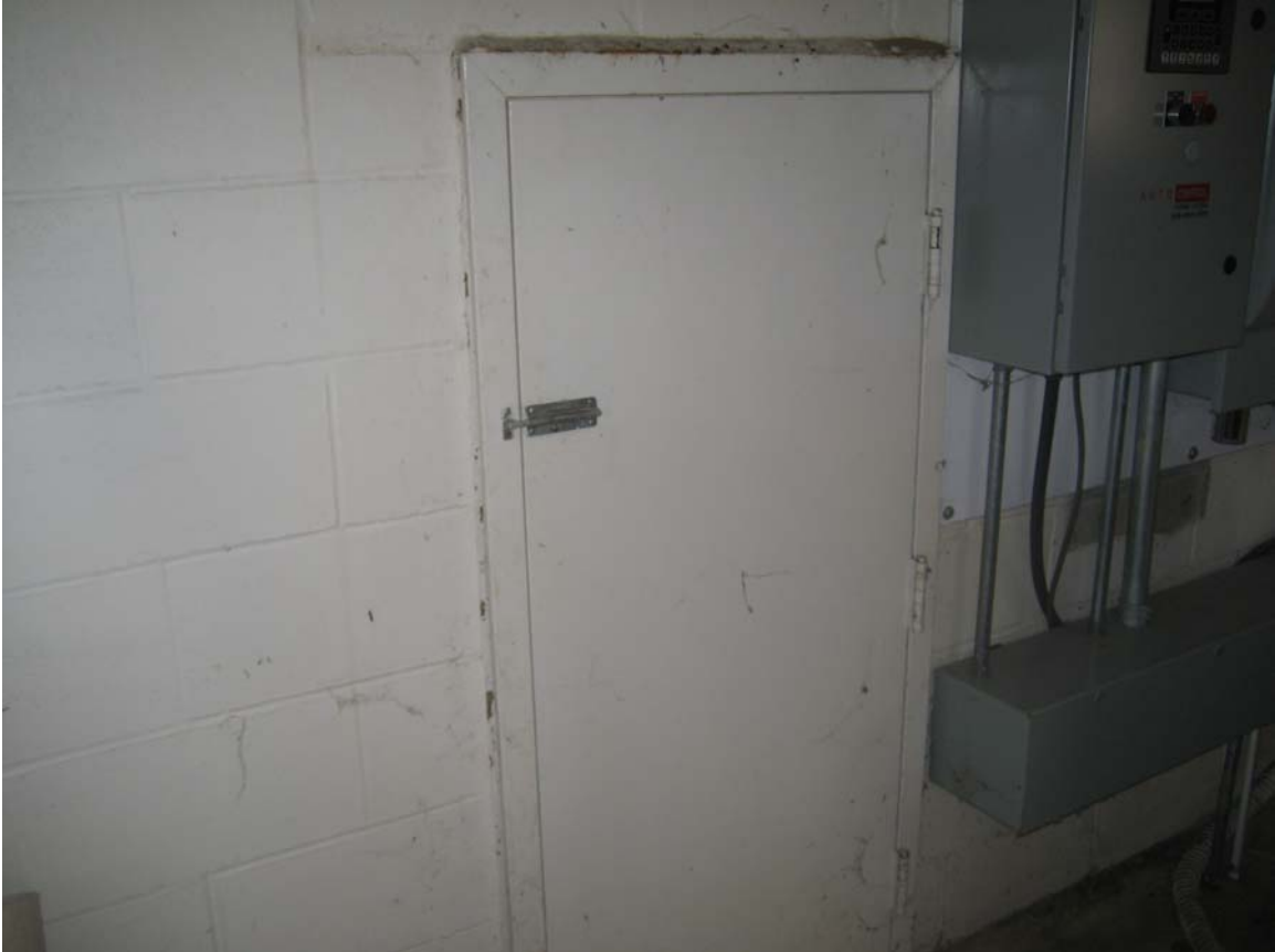
HA #1 – Assumed Fire Door and Frame
