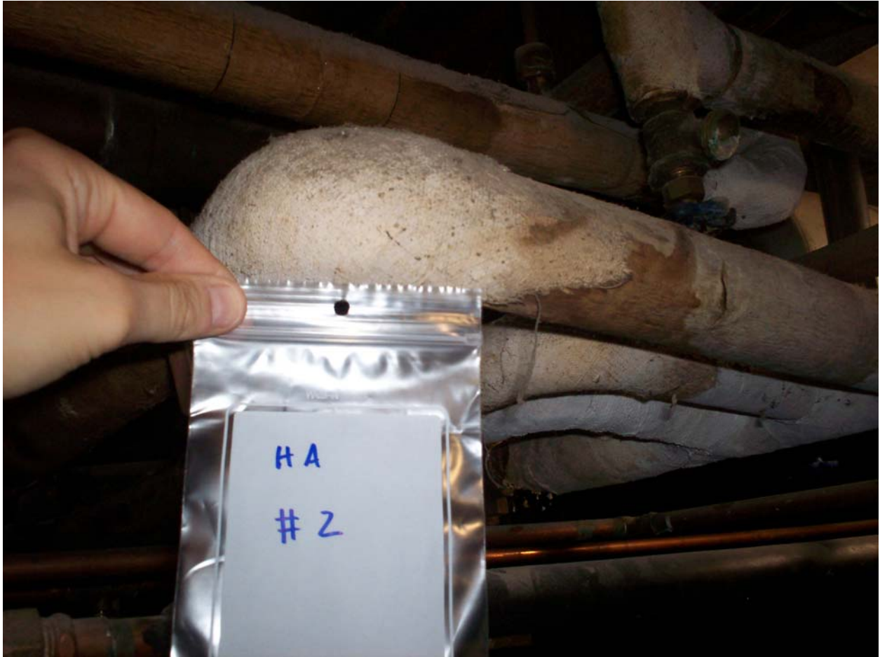
HA #2 – Asbestos containing domestic water supply pipe joint and hanger insulation
