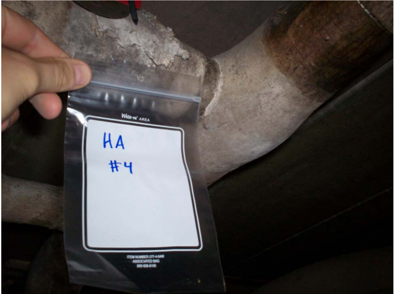
HA #4 – Asbestos containing steam/condensate pipe joint and hanger insulation
