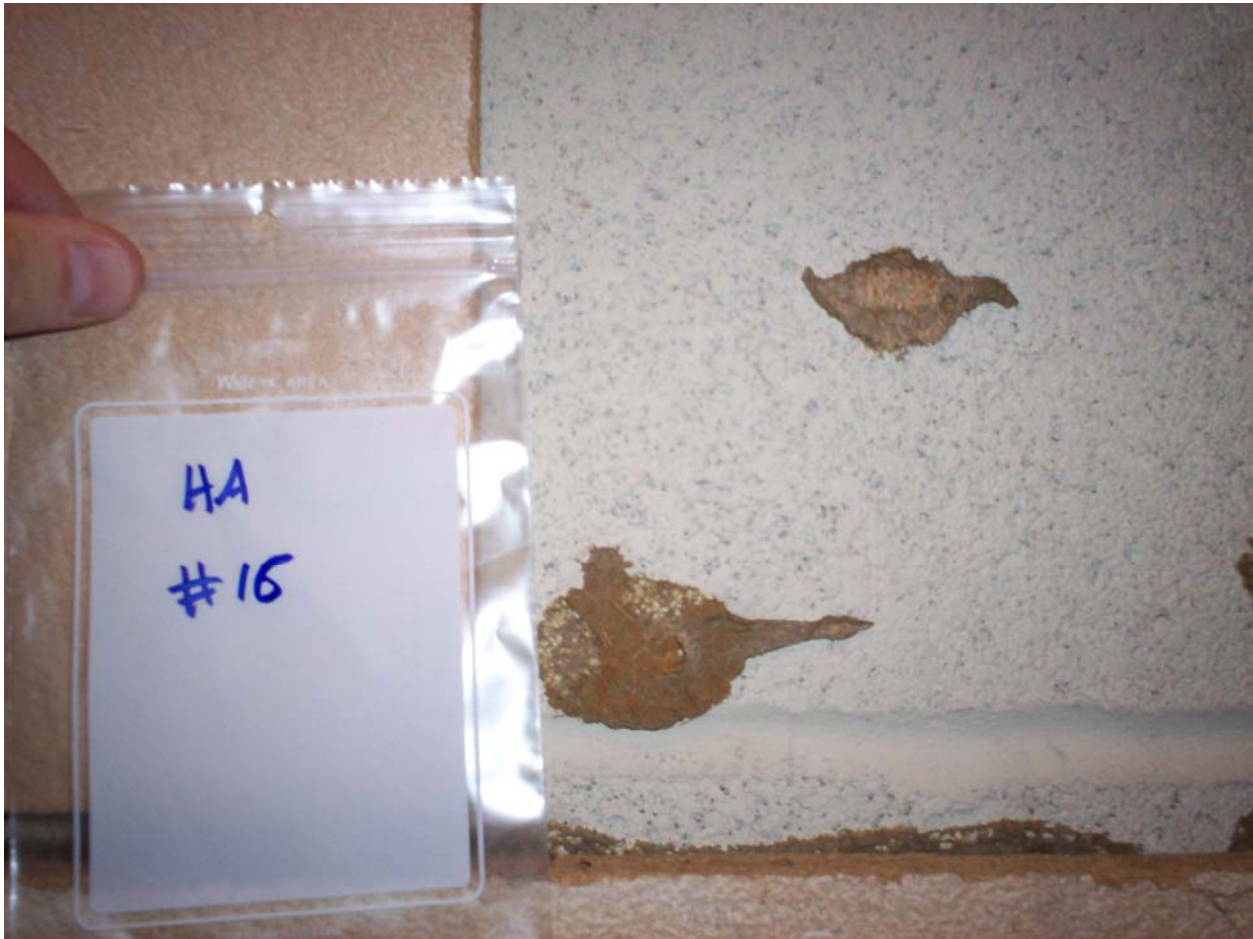
HA #16 – Asbestos containing wallboard glue pods
