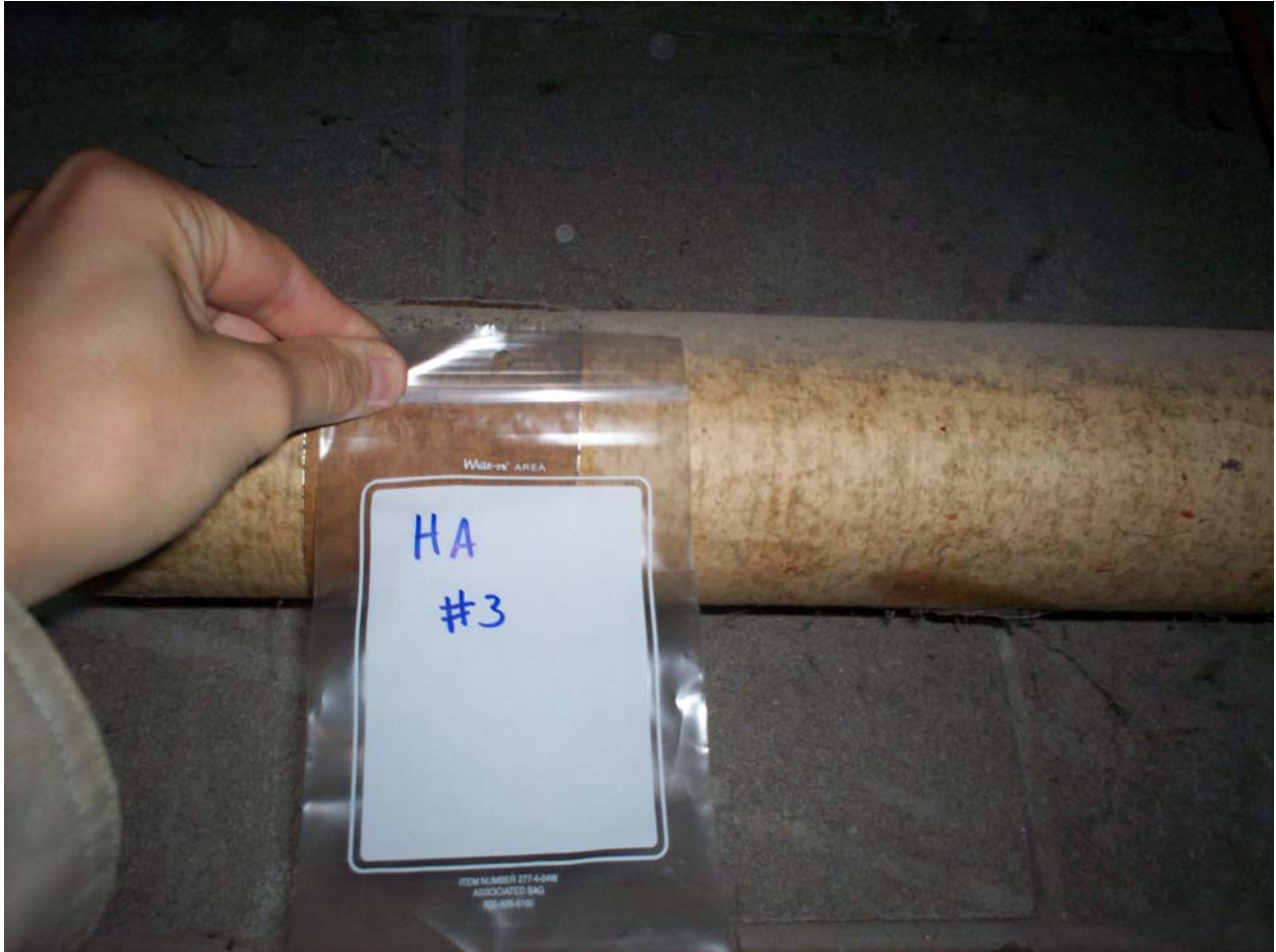
HA #3 – Non asbestos containing steam/condensate pipe straight insulation (fiberglass) wrap
