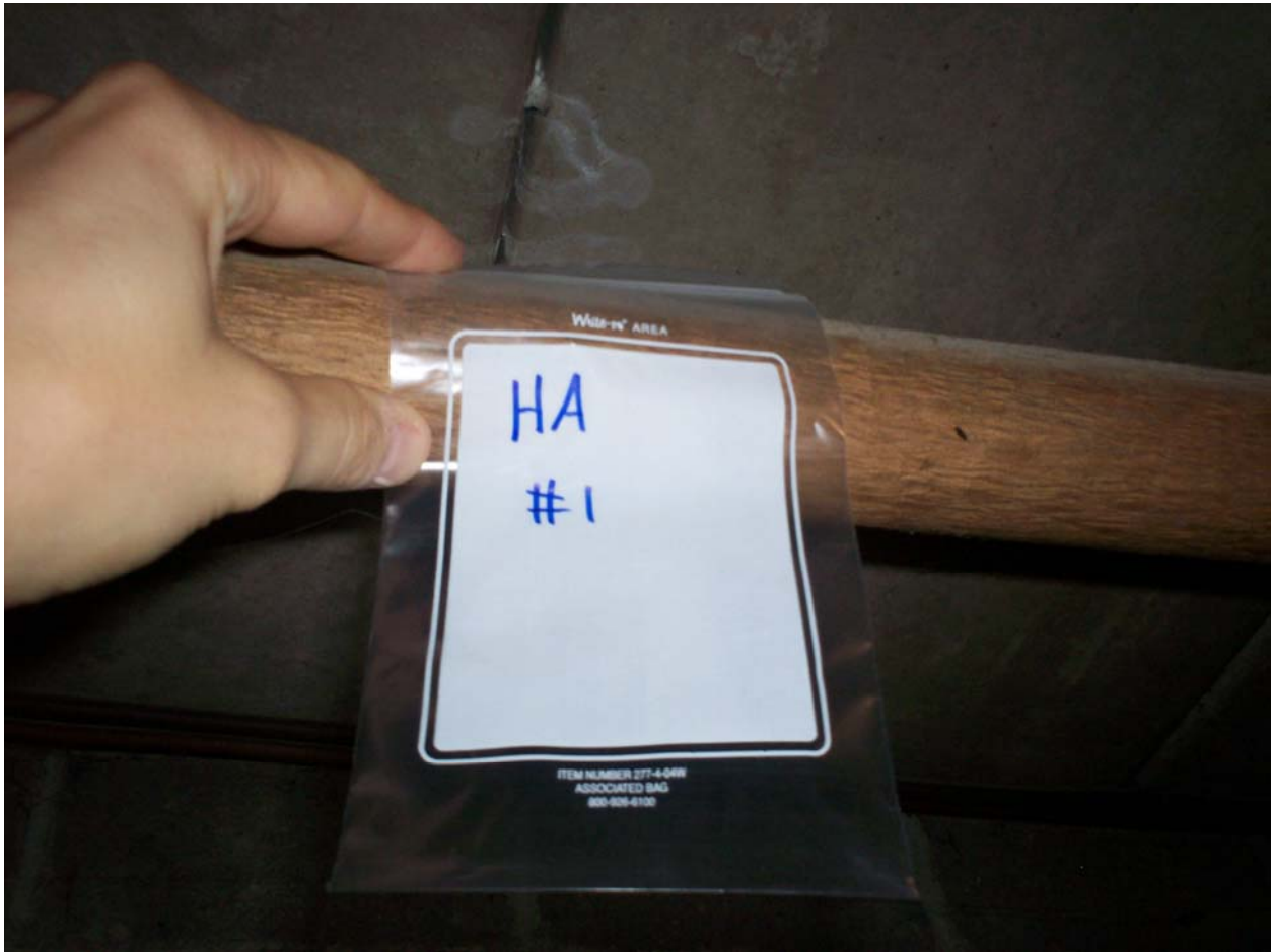
HA #1 – Non asbestos containing domestic water supply pipe straight insulation (fiberglass) wrap
