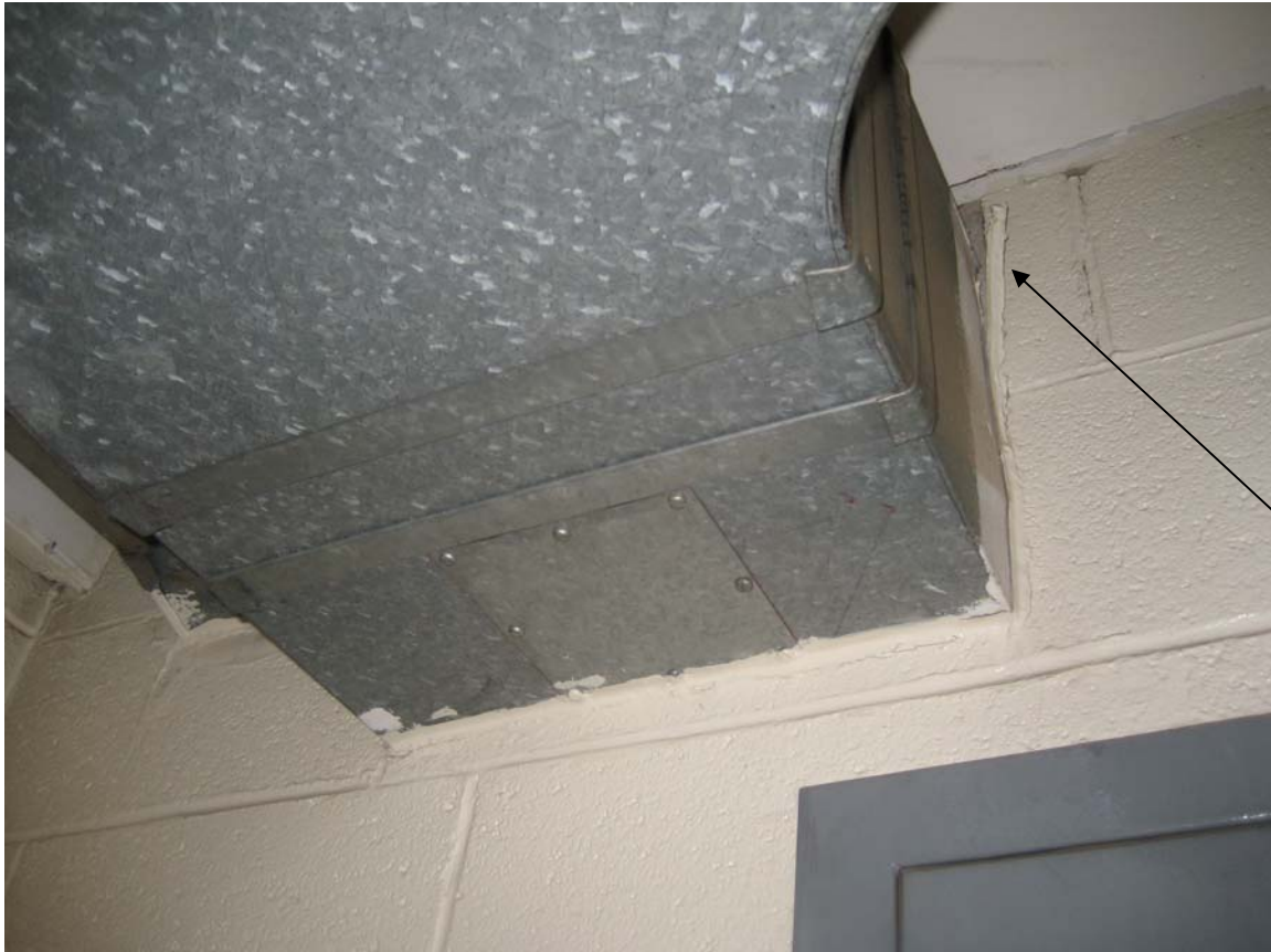
HA #5 – Non asbestos containing white caulk around duct
