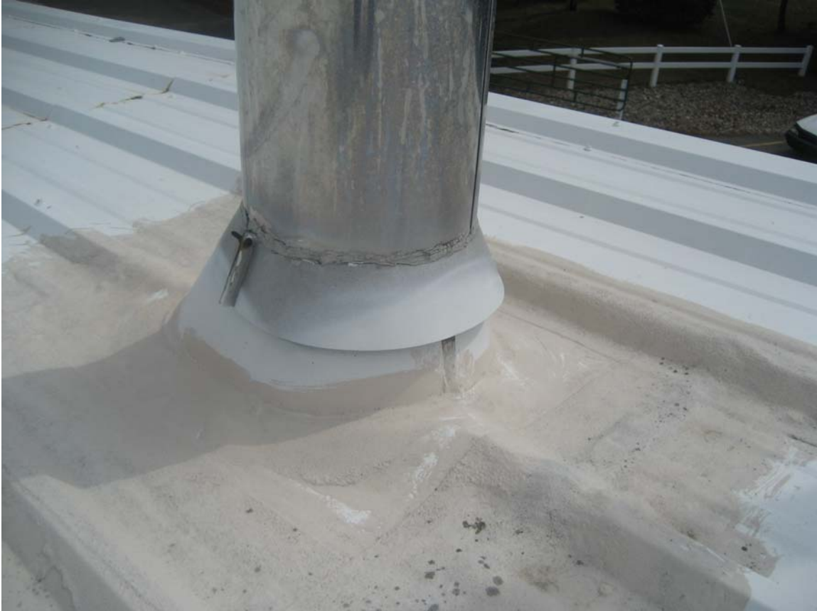
HA #9 – Assumed asbestos containing roofing caulk
