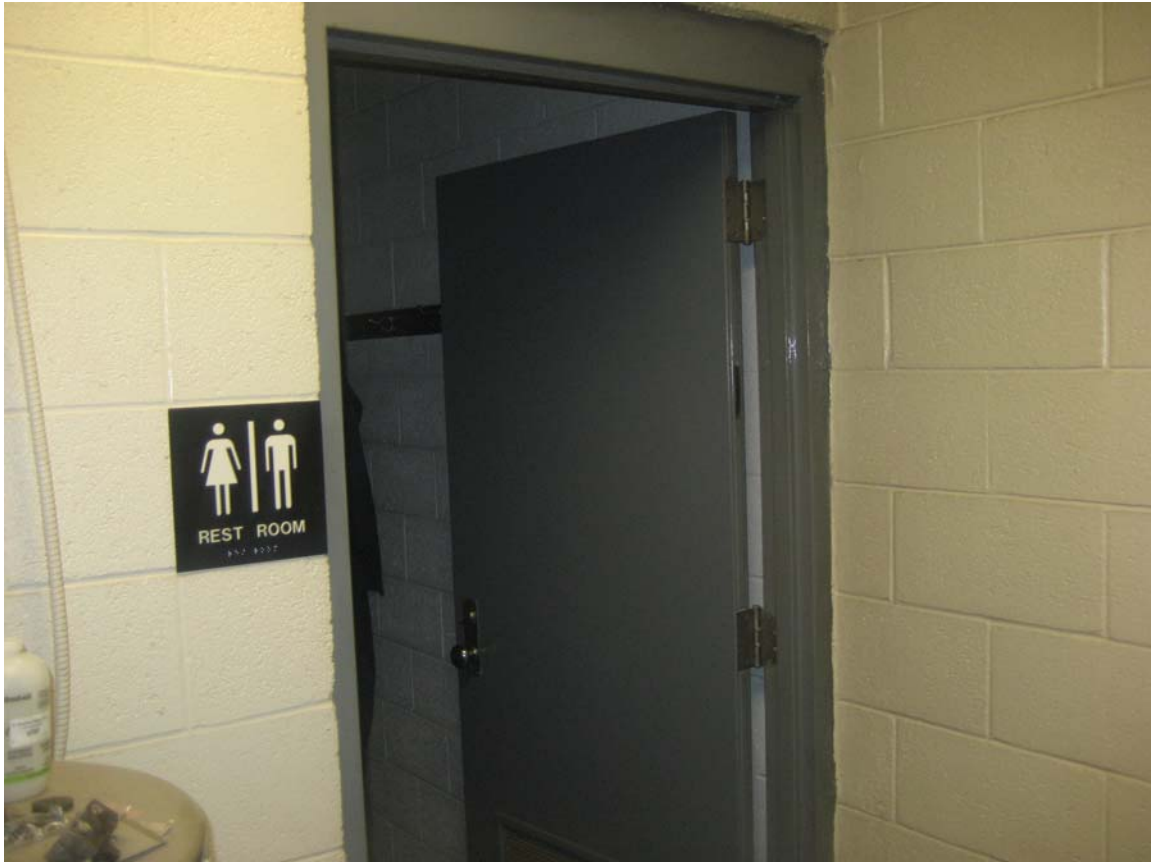
HA #8 – Assumed asbestos containing fire door and frame
