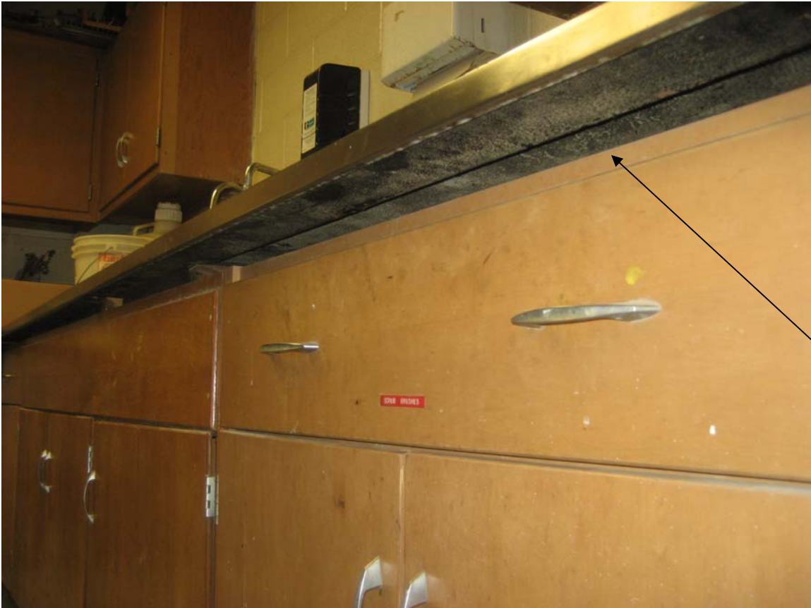
HA #3 – Asbestos containing sink and lab bench undercoating
