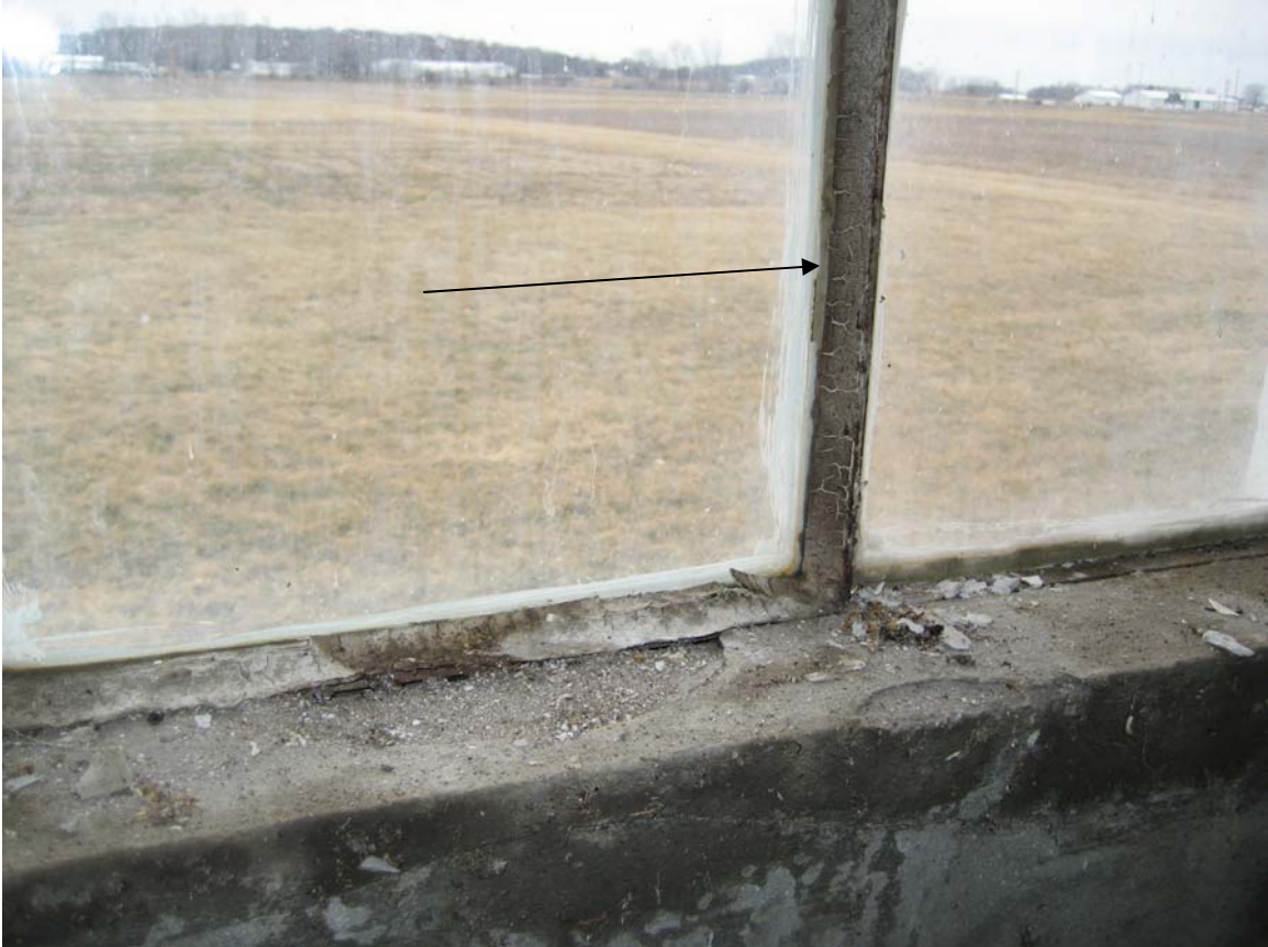
HA #1 – Non-asbestos containing white window glazing
