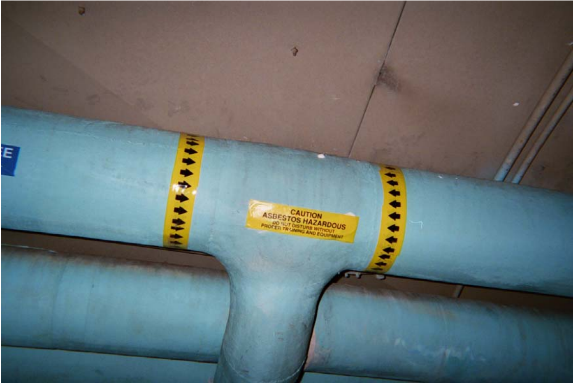
Photo 2 – Asbestos-containing domestic water pipe joint insulation
