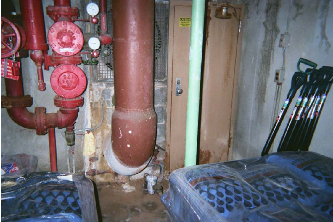
Photo 1 – Asbestos-containing steam/condensate pipe joint insulation
