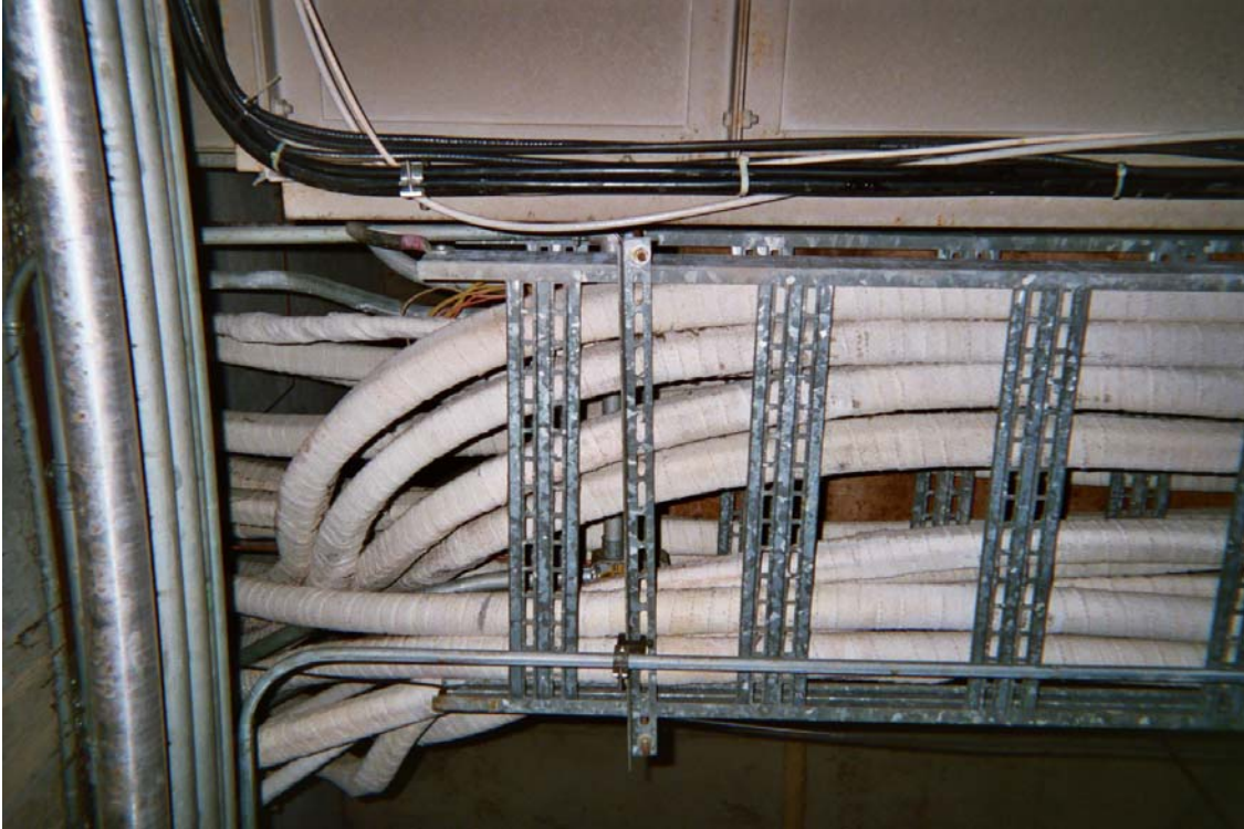
Photo 11 – Asbestos-containing electrical insulation cloth
