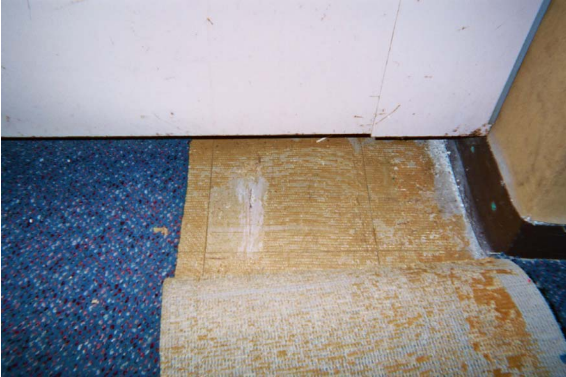
Photo 13 – Asbestos-containing 9” x 9” light brown floor tile with cream and rust streaks and associated mastic
