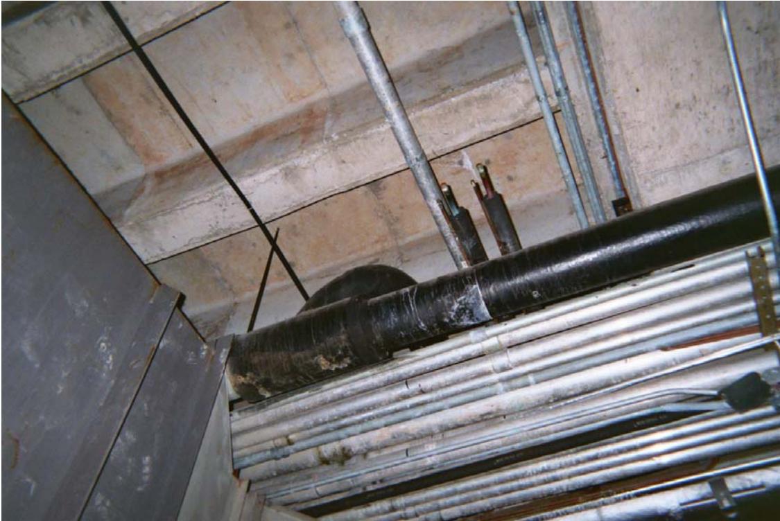
Photo 4 – Asbestos-containing sewer drain pipe joint insulation
