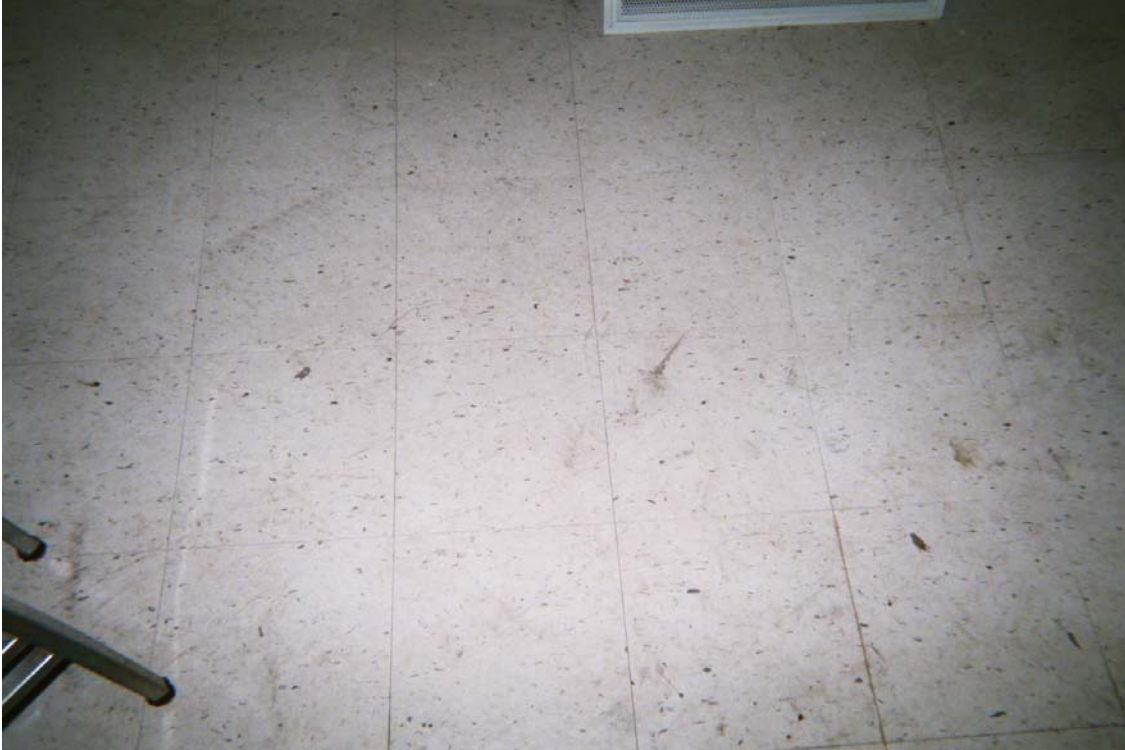
Photo 12 – Non-asbestos containing 12” x 12” light cream floor tile with gray specks and associated mastic
