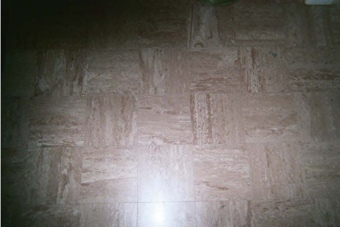
Photo 5 – Asbestos-containing 9” x 9” beige floor tile with swirls and associated mastic
