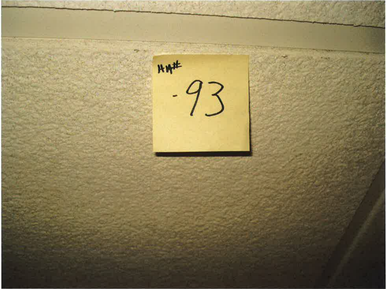
HA #93 – Non asbestos containing 2' x 2' white drop-in ceiling tile with rough texture
