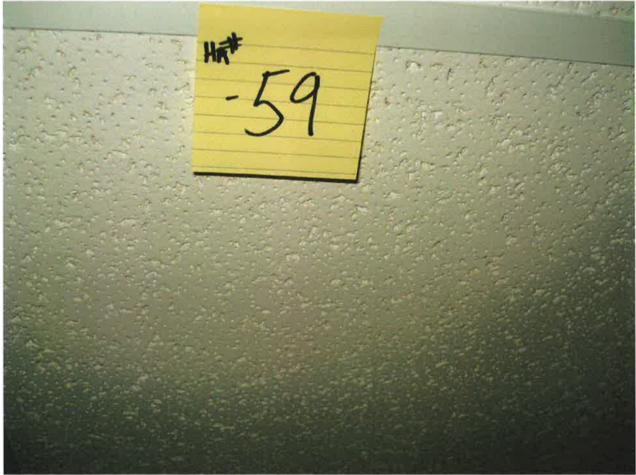
HA #59 – Non asbestos containing 2' x 2' white lay-in ceiling tile with pin holes and random gouge pattern
