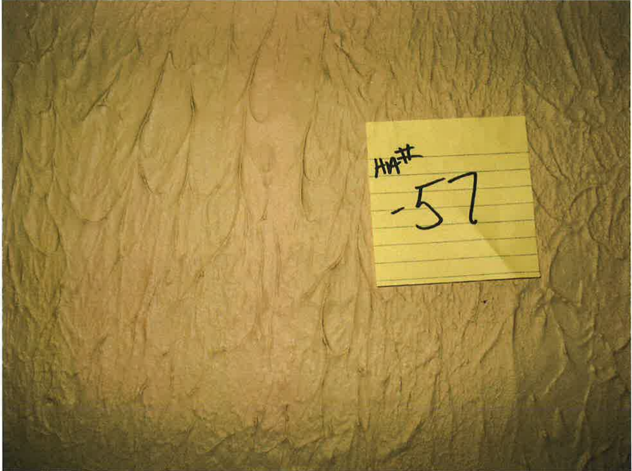
HA #57 – Non asbestos containing heavy textured wall plaster
