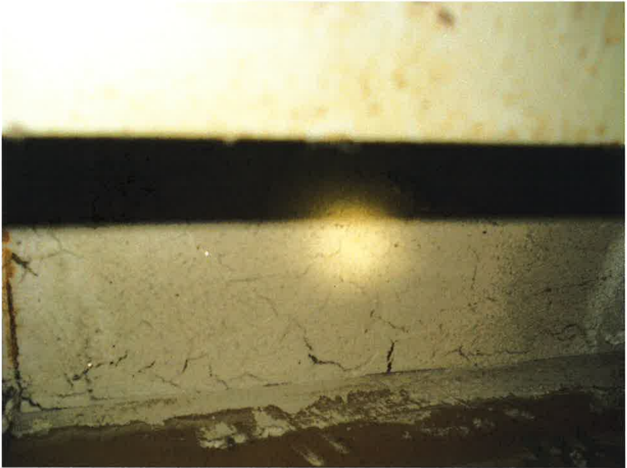
HA #99 – Asbestos containing troweled on beam material (white)
