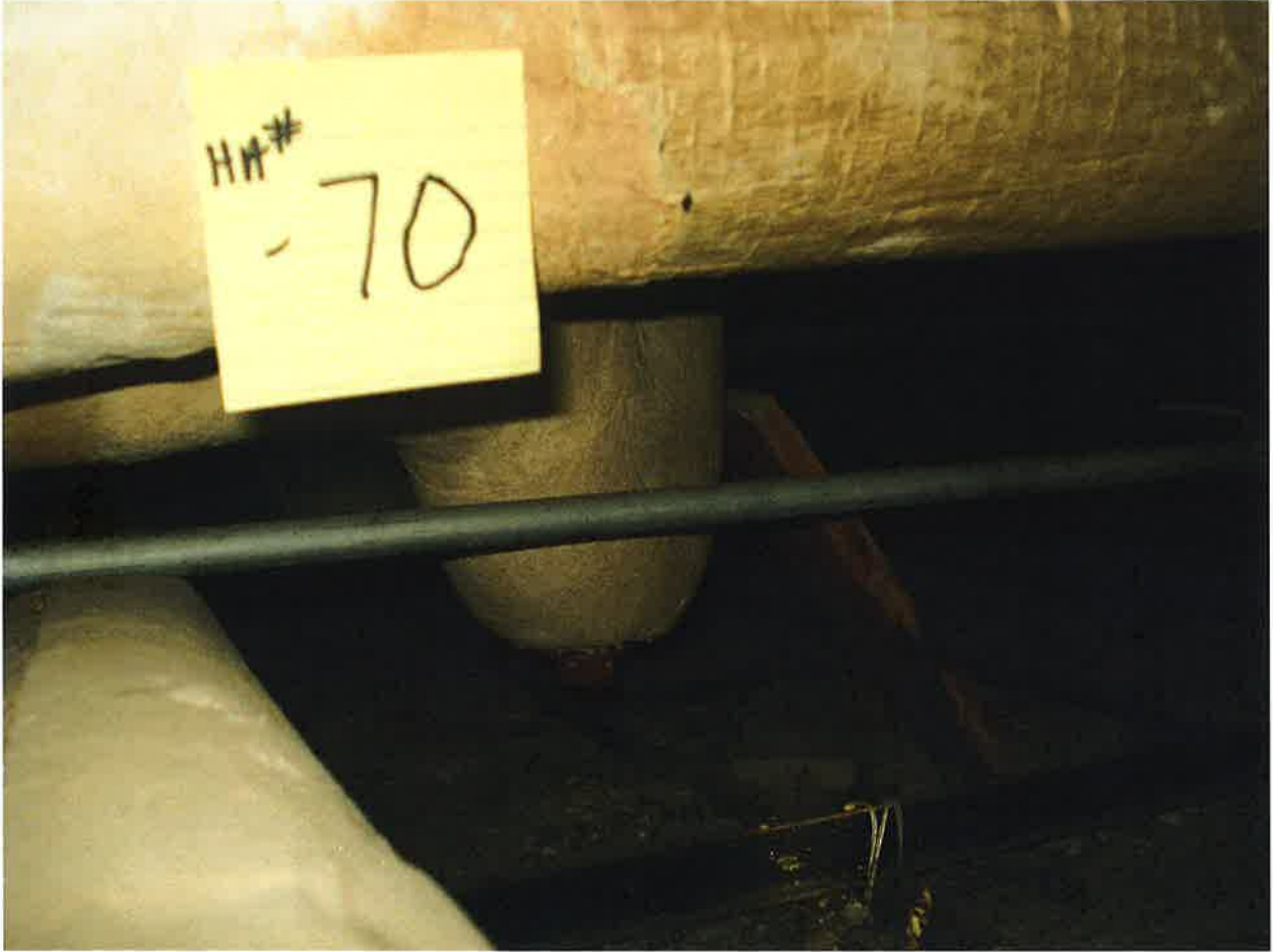
HA #70 – Asbestos containing drain line pipe joint and hanger insulation
