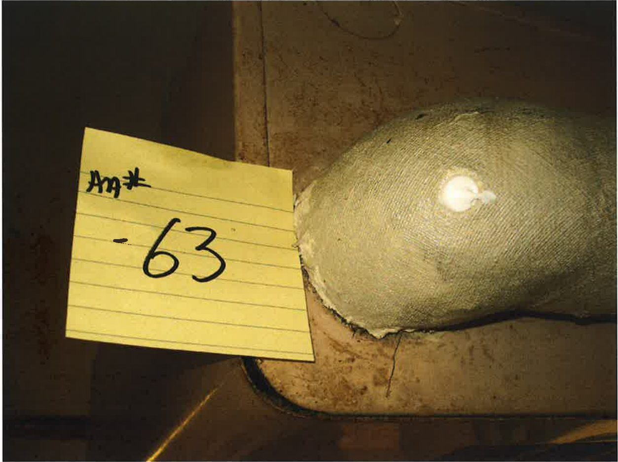
HA #63 – Non asbestos containing hot heating water supply pipe joint and hanger insulation
