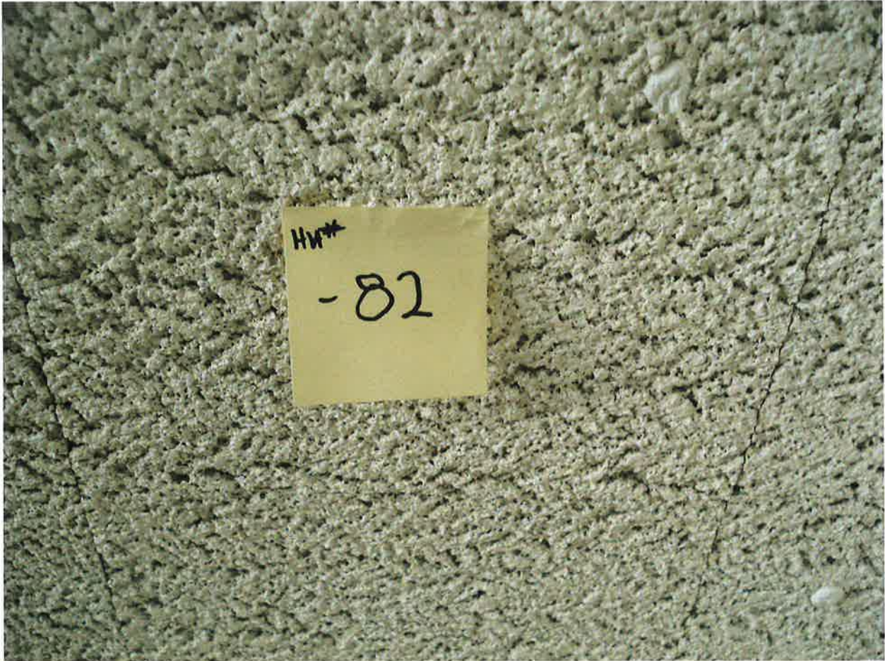
HA #82 – Non asbestos containing 12” x 12” white ceiling tile with deep texture and associated glue pods
