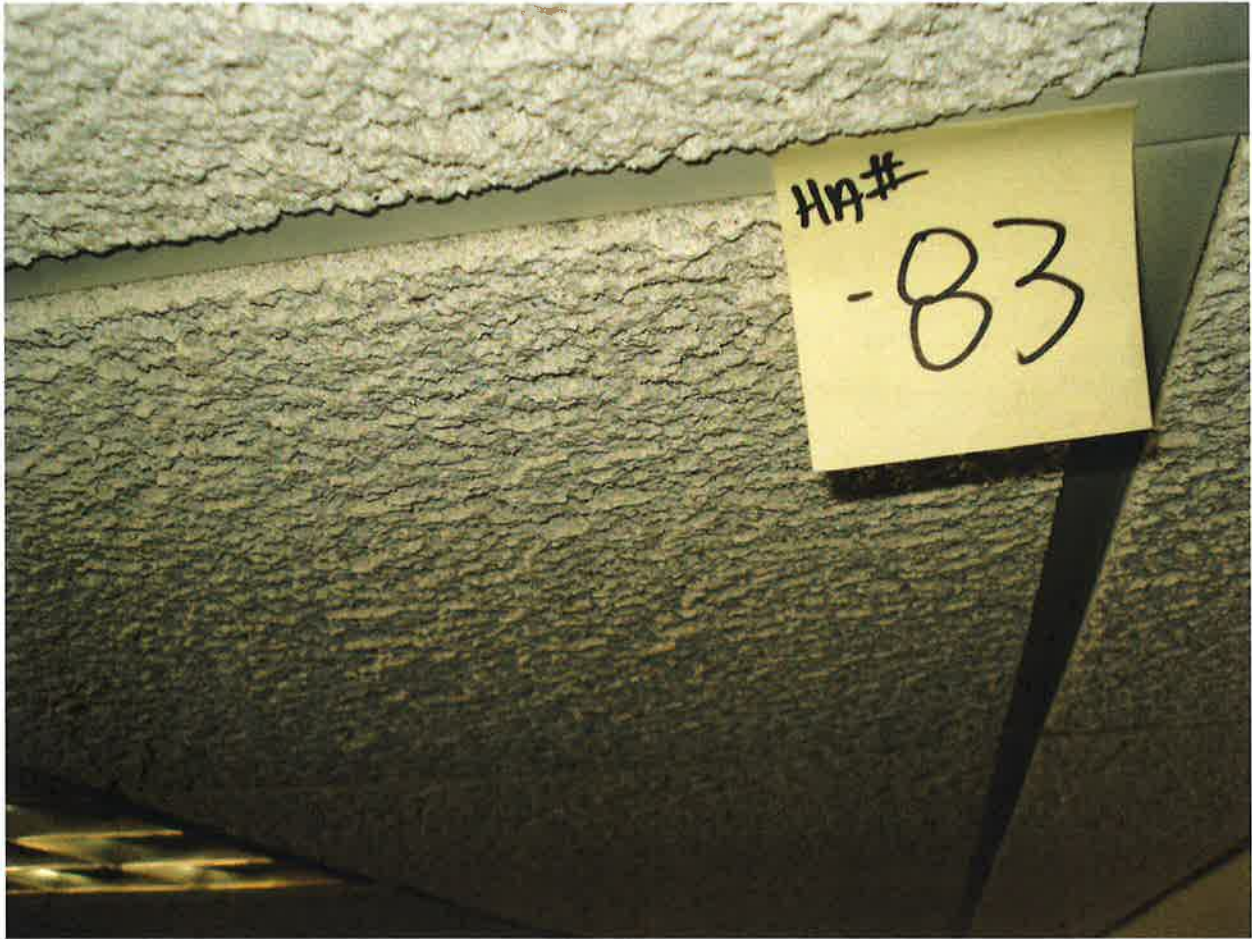
HA #83 – Non asbestos containing 2' x 2' white drop-in ceiling tile with deep texture
