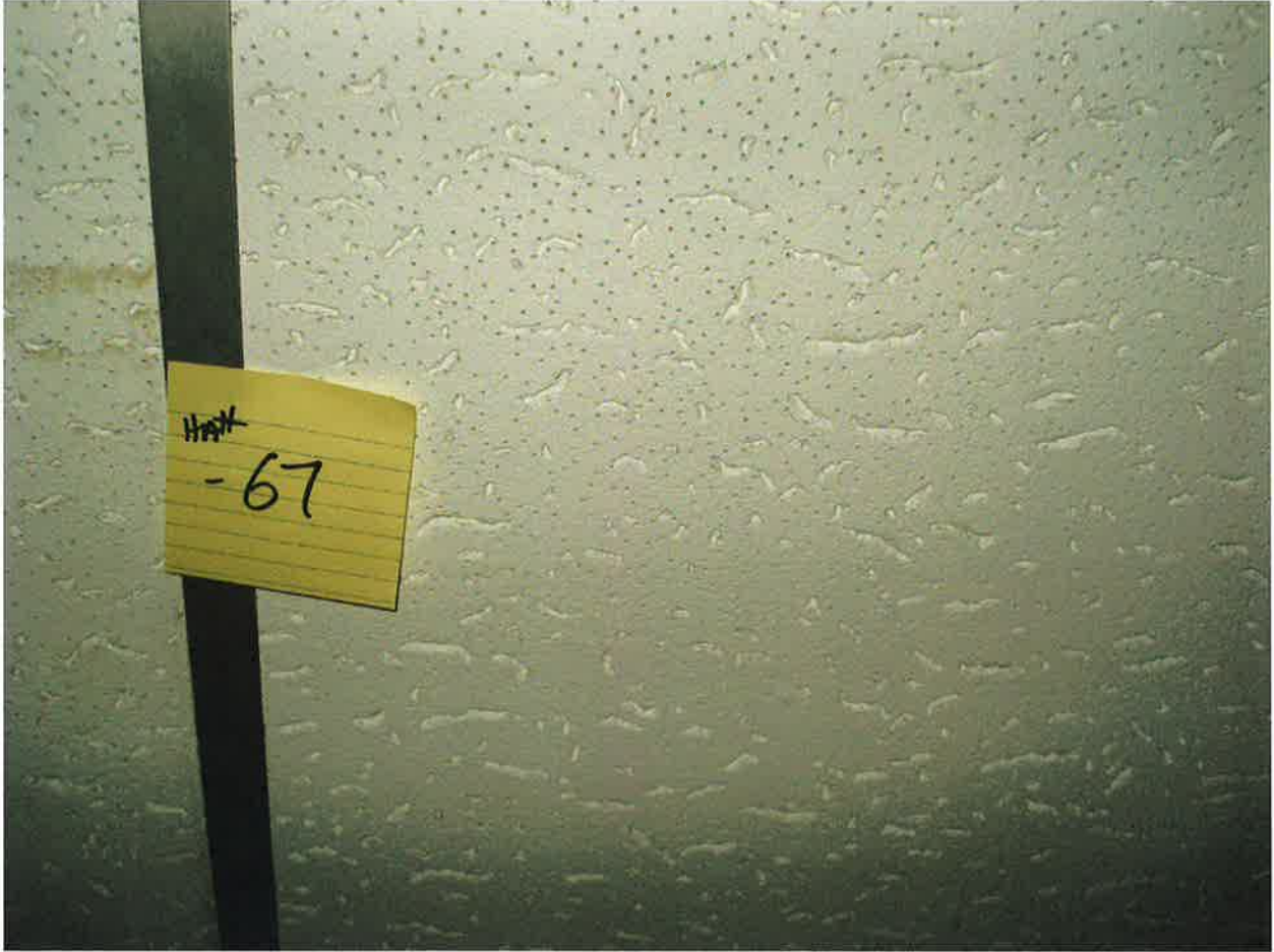
HA #67 – Non asbestos containing 2' x 4' white lay-in ceiling tile with pin holes and fissures
