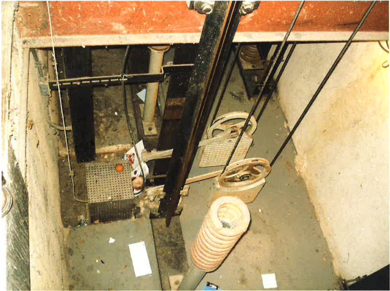
North central elevator cable system
