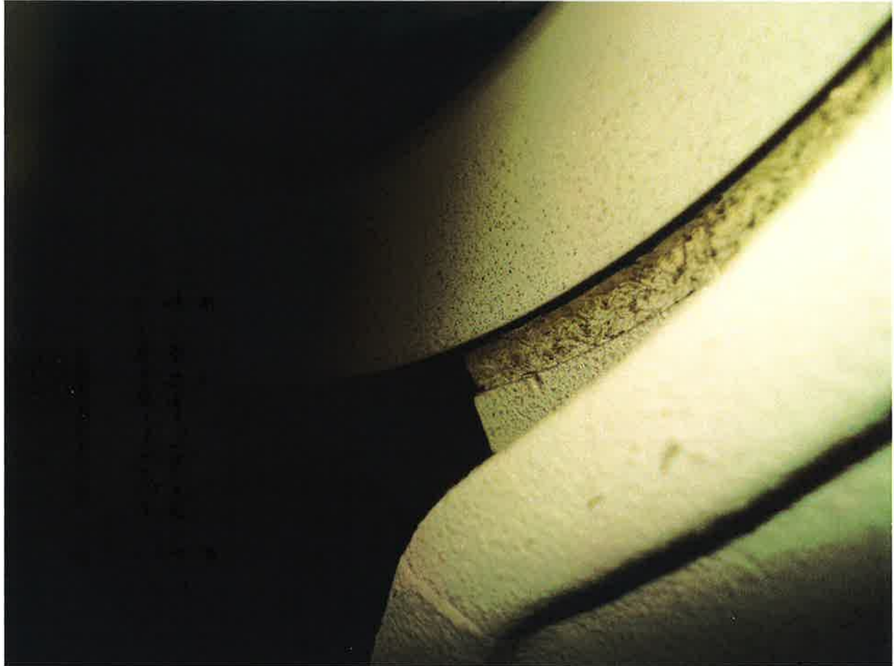
HA #89 – Assumed asbestos-containing freight elevator brake
