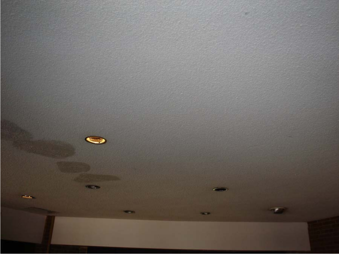
Photo 1 – Asbestos-containing spray-on acoustical ceiling plaster (popcorn)
