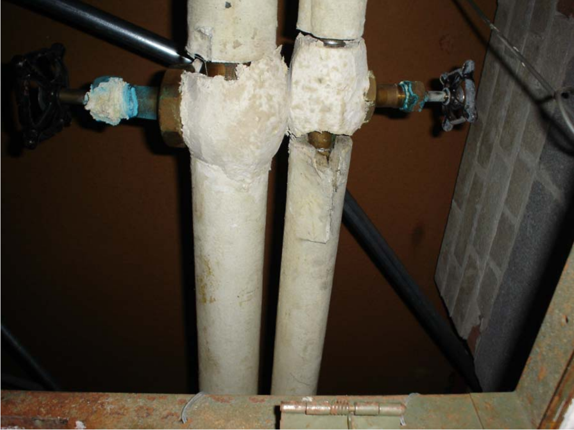
Photo 15 – Asbestos-containing steam/condensate supply and return pipe straight, pipe joint and hanger insulation
