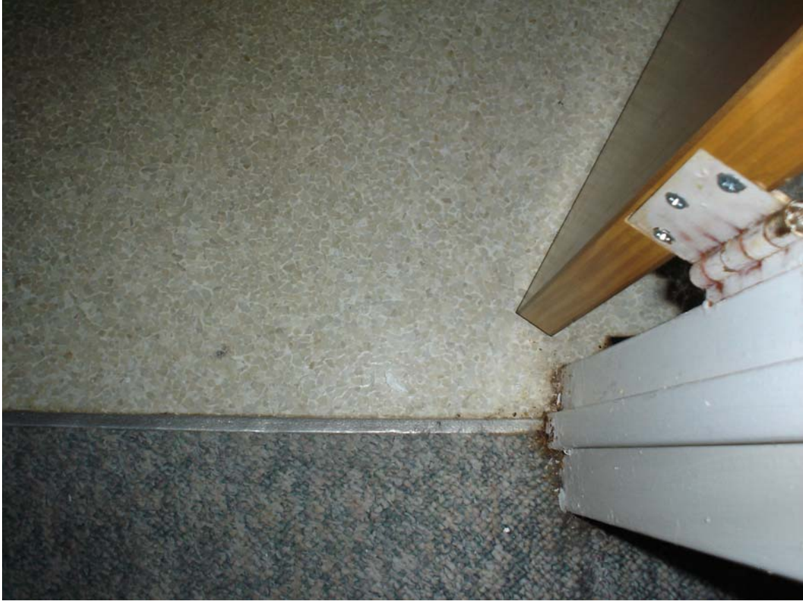
Photo 6 – Asbestos-containing cream linoleum with mosaic pattern and associated mastic
