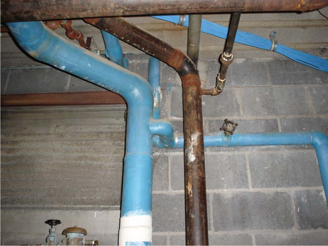
Photo 7 – Non asbestos-containing domestic water supply and return pipe joint and hanger insulation and Asbestos-containing domestic water supply and return pipe straight insulation
