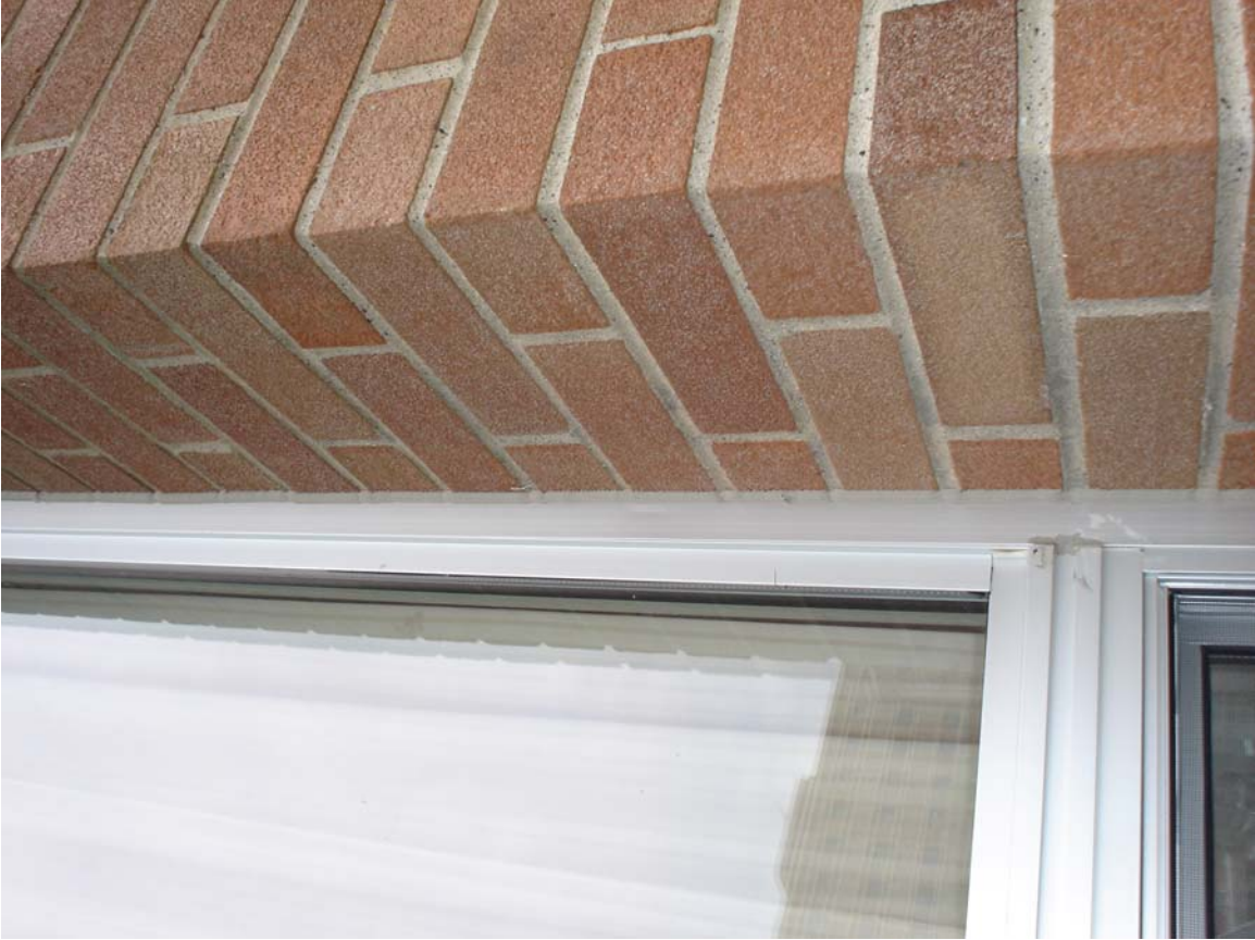
Photo 12 – Assumed asbestos-containing window and door frame caulk compound
