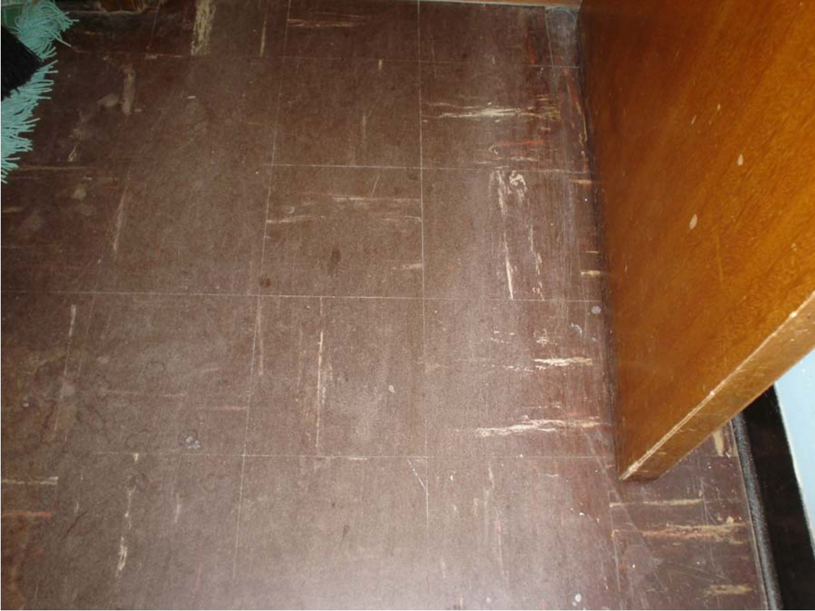
Photo 14 – Asbestos-containing 9” x 9” dark brown floor tile with cream and rust streaks and associated mastic
