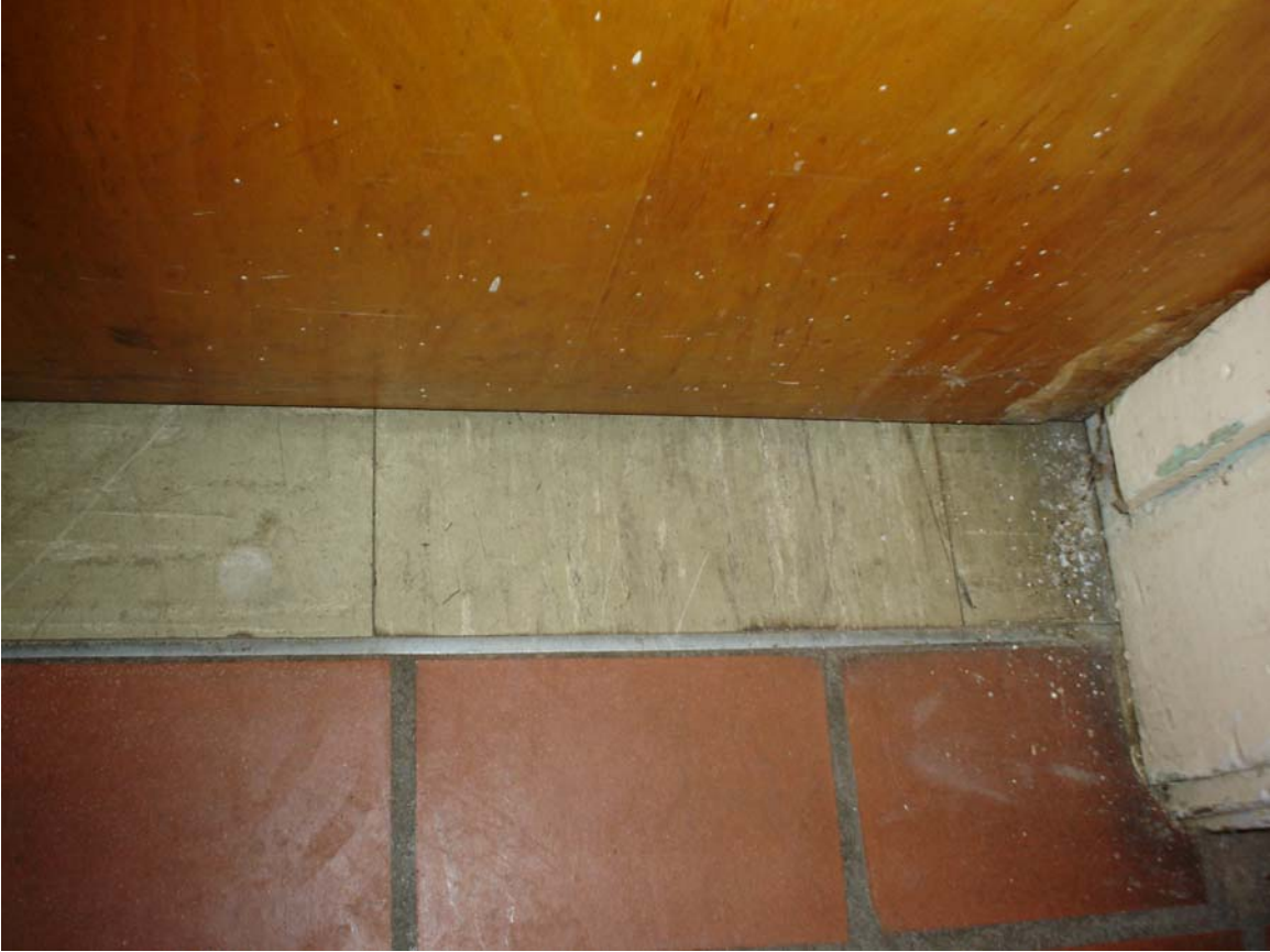
Photo 11 – Asbestos-containing 9” x 9” beige floor tile with cream and tan streaks and associated mastic
