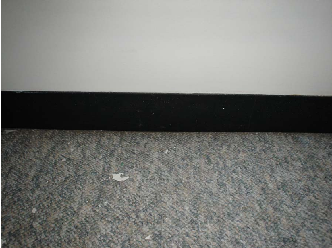
Photo 3 – Non asbestos-containing 4” black cove molding and associated mastic
