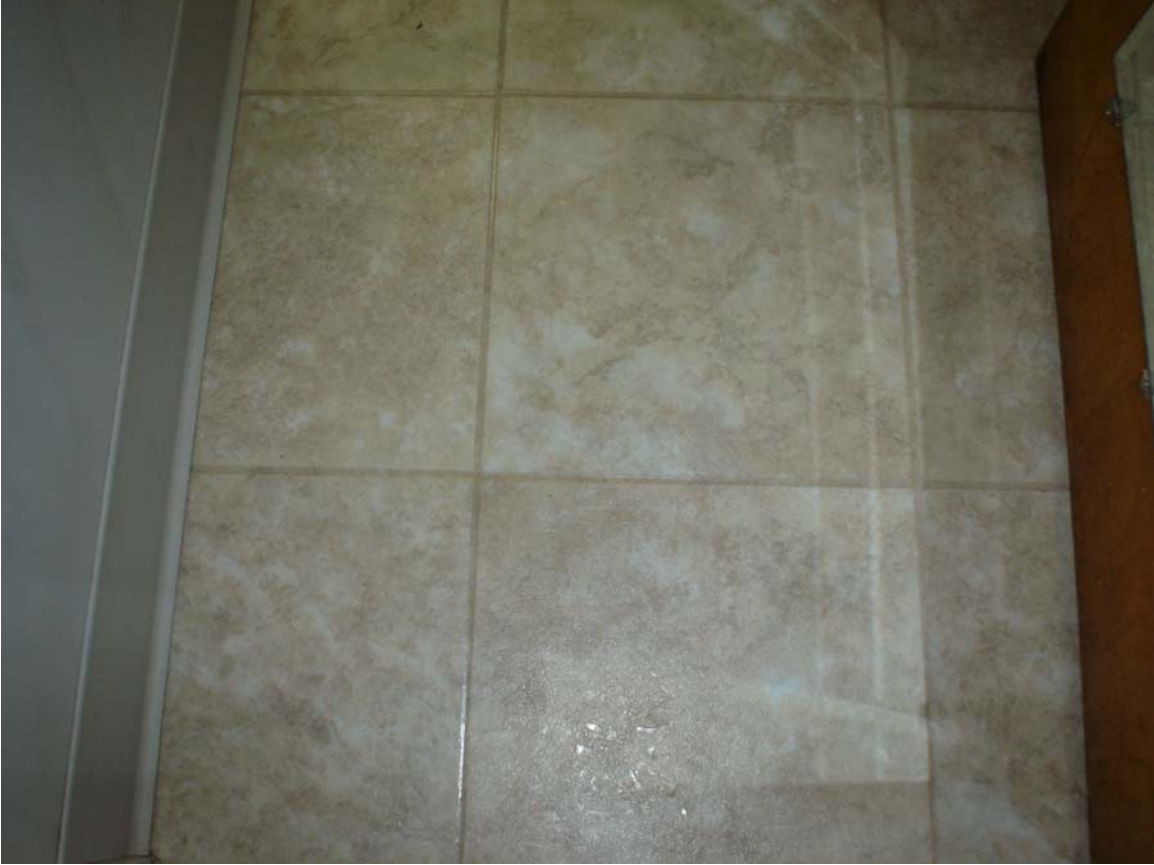
Photo 8 – Non asbestos-containing 12” x 12” tan linoleum with swirl pattern and associated mastic and Non asbestos-containing 4” cream cove molding and associated mastic
