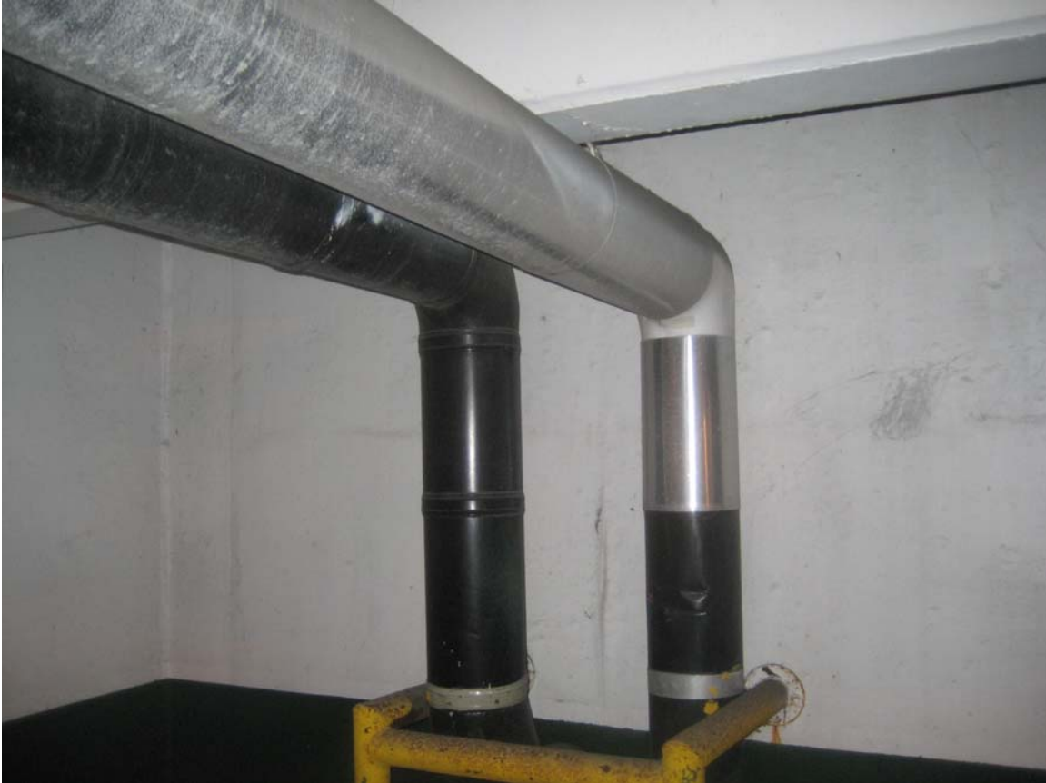
HA #7 – Asbestos containing metal jacketed steam supply and return lines
