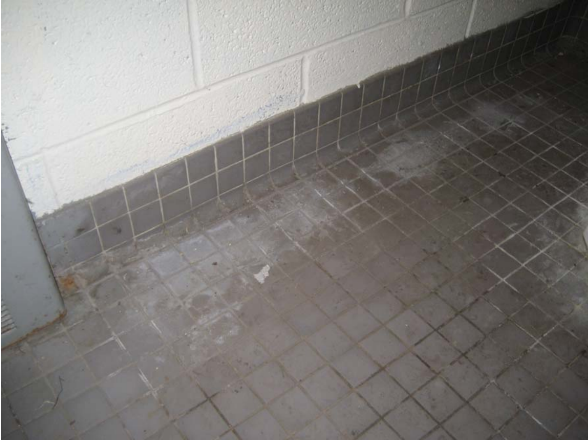
HA #4 – Asbestos containing 2”x 2” Grey ceramic tile and associated bedding compound
