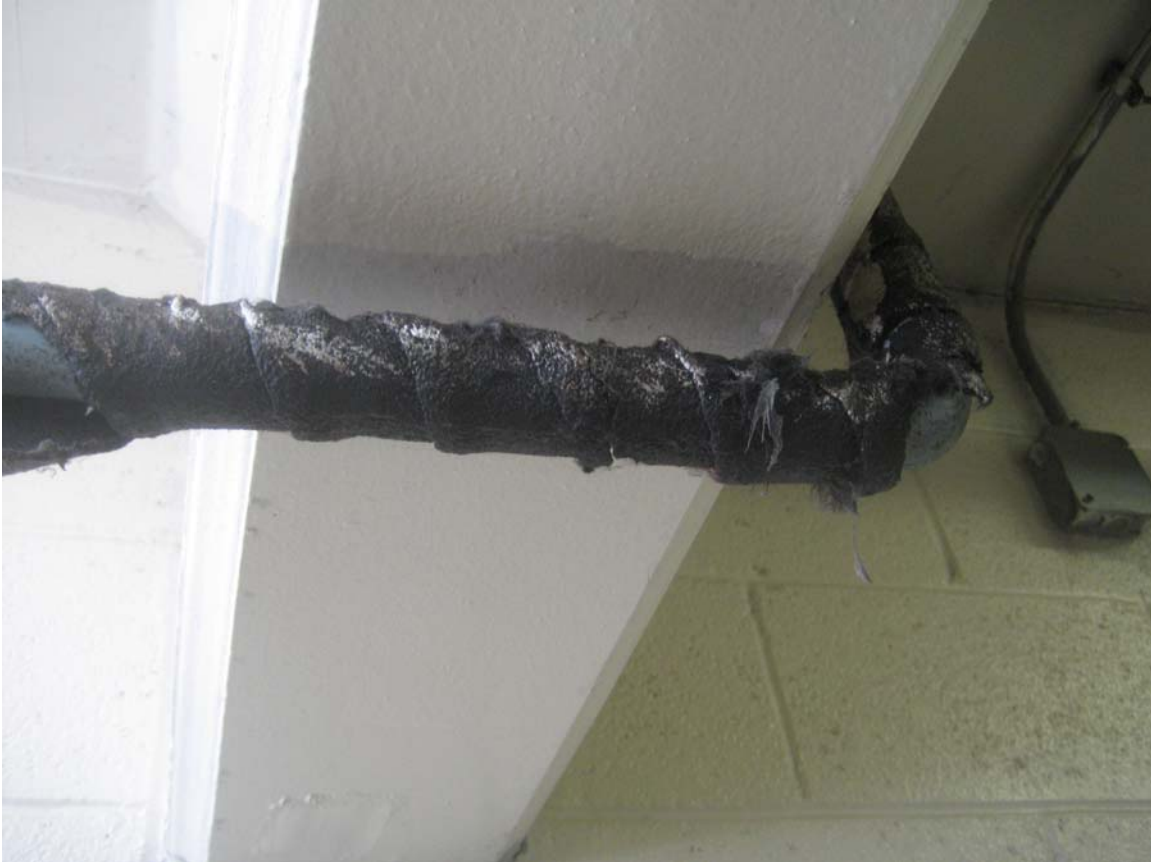
HA #1 – Asbestos containing Black Pipe Wrap
