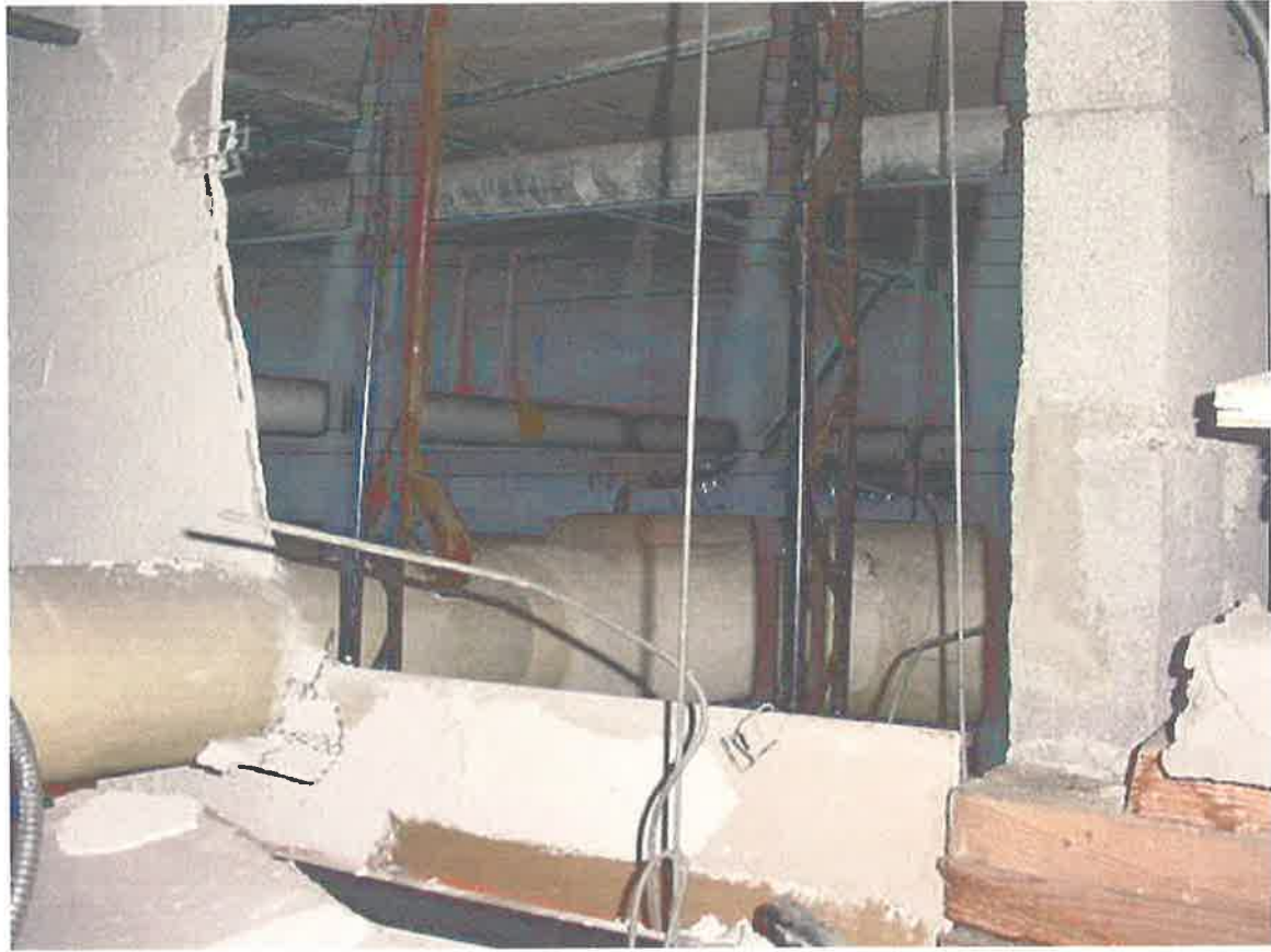
Photo 31 – Fire protection ceiling board in 5 th floor ceiling access area
