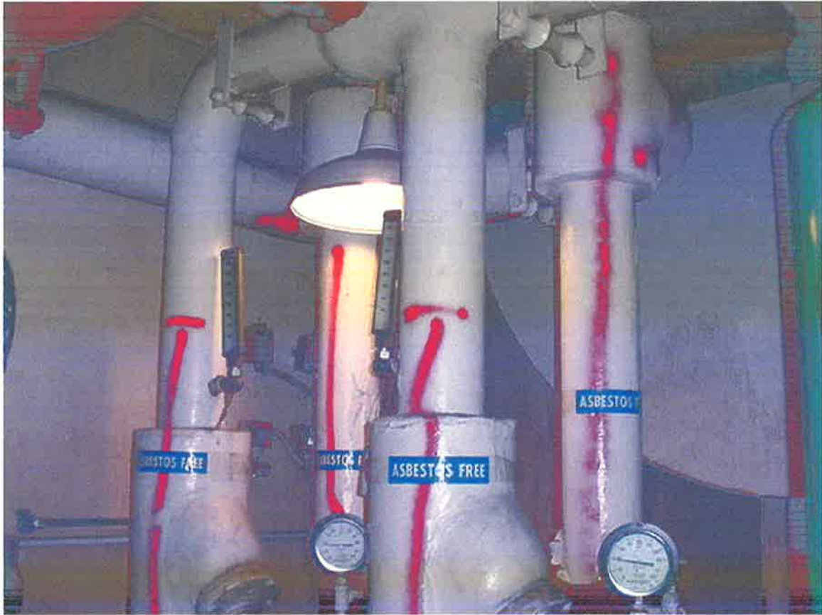
Photo 22 - Mechanical room 50, white chilled water pipe joint insulation, northeast of tunnel entrance
