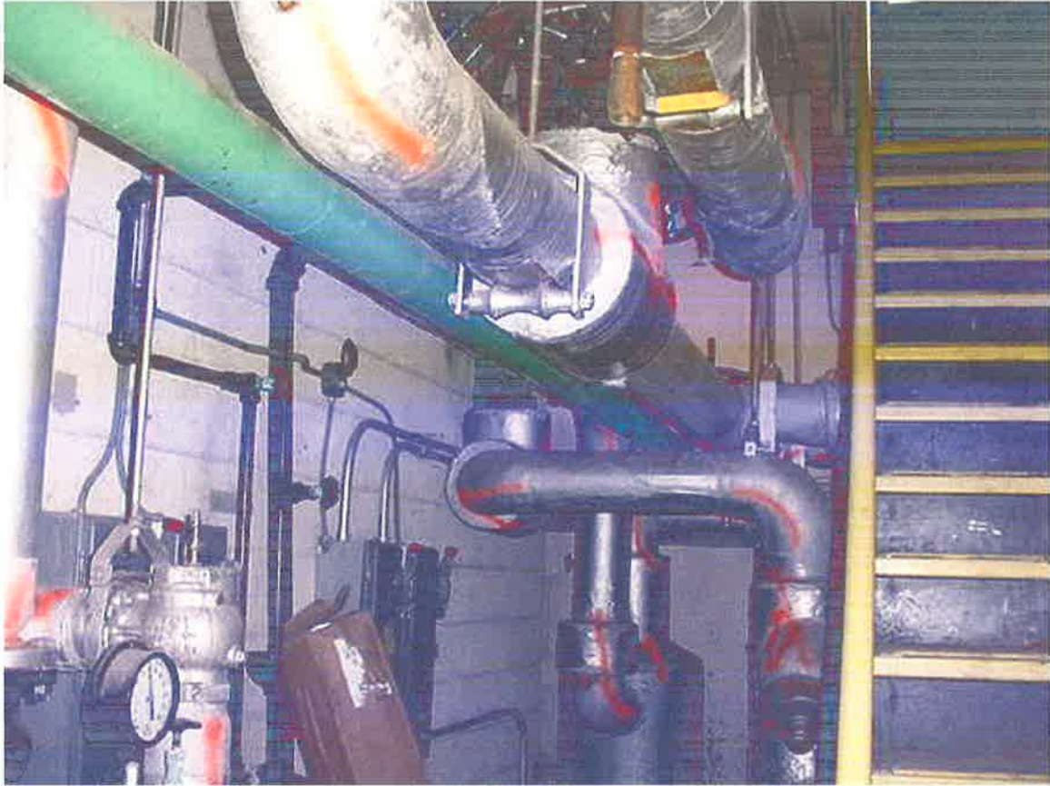
Photo 19 – Mechanical Room 50, silver treated pipe joint insulation
