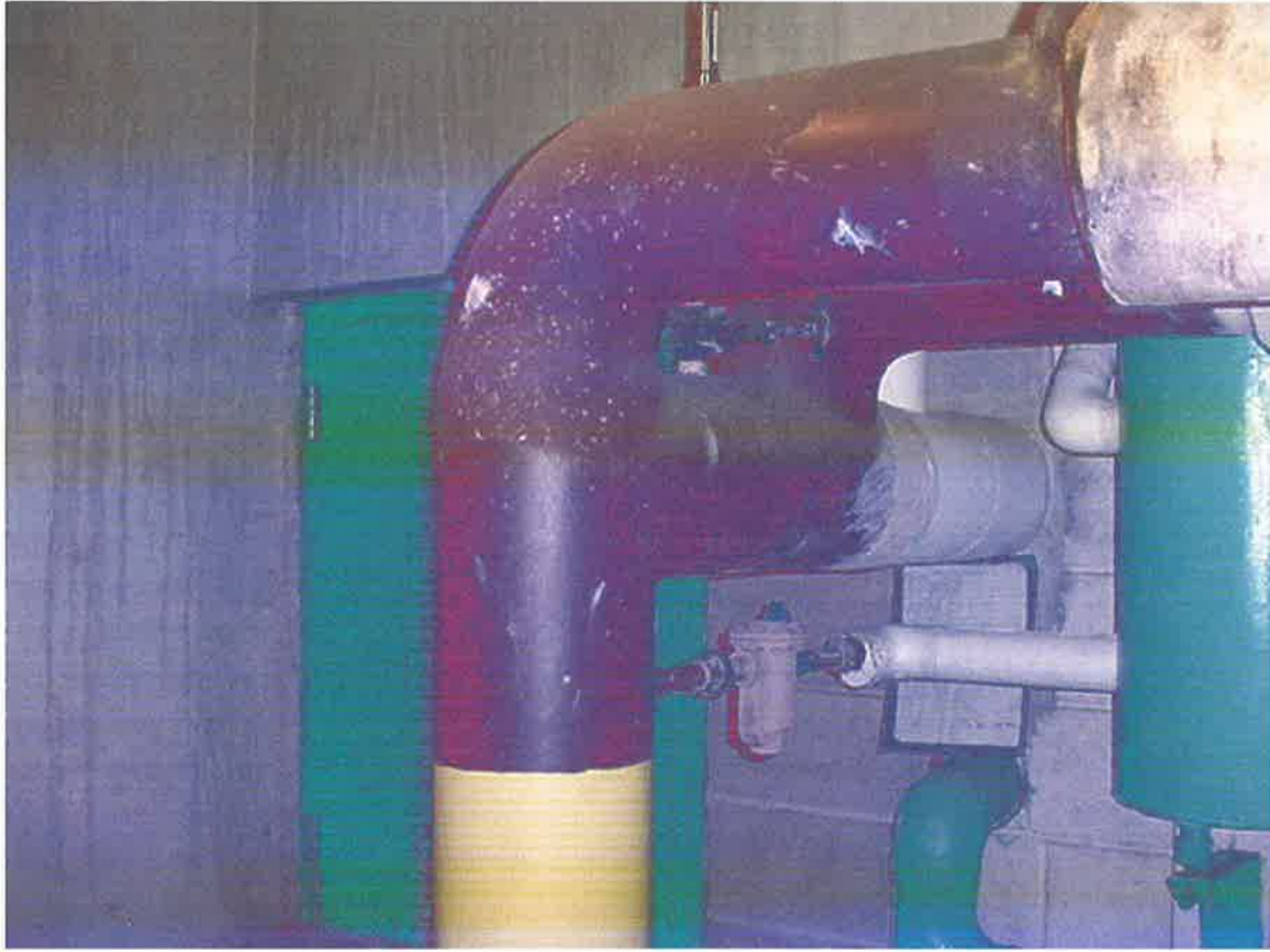
Photo 20 – Mechanical room 50, maroon high pressure steam pipe straight insulation and pipe joint insulation, southwest of tunnel access
