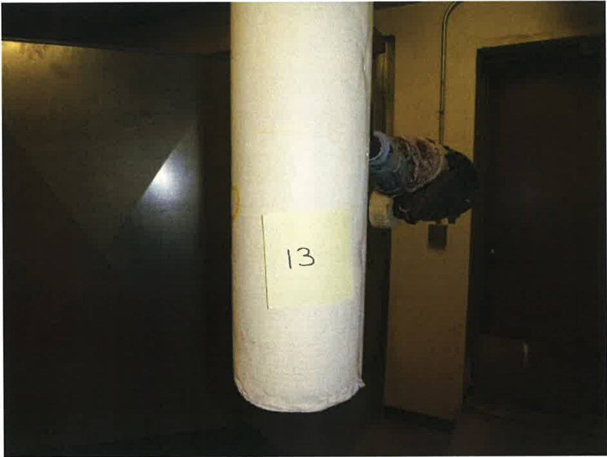
Chemistry Building HA 13 Fiberglass Pipe Insulation - New Non-Asbestos
