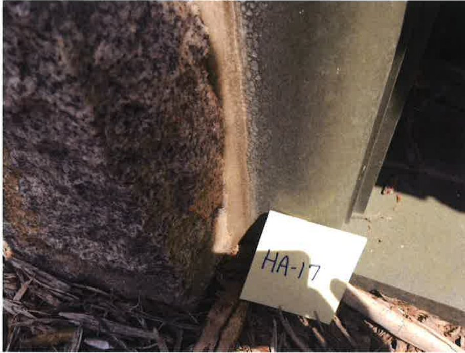
HA-17 Non-asbestos containing exterior green window caulk
