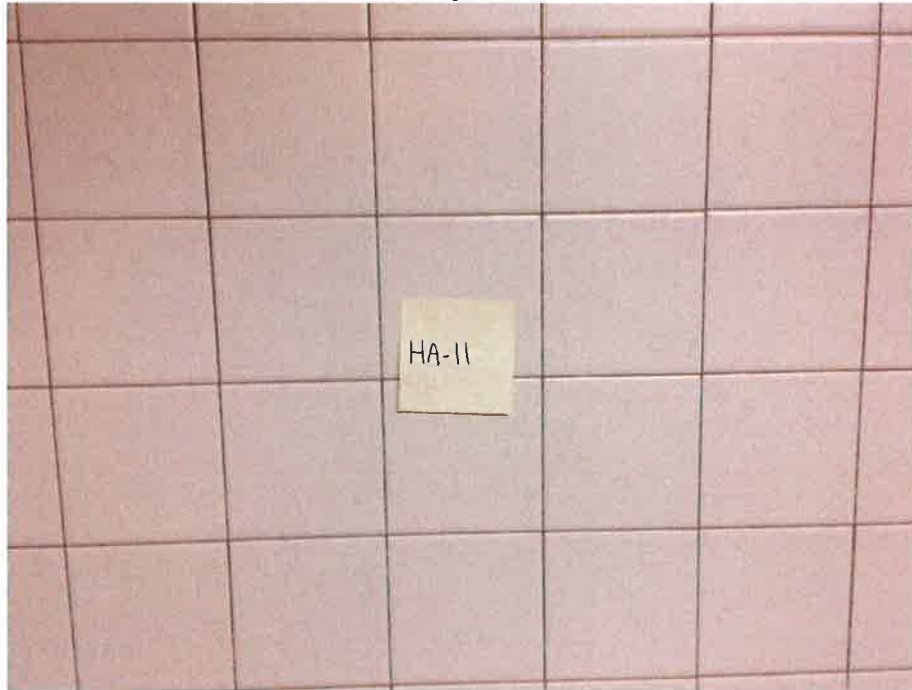
HA-11 Assumed asbestos-containing ceramic wall tile bedding compound and grout
