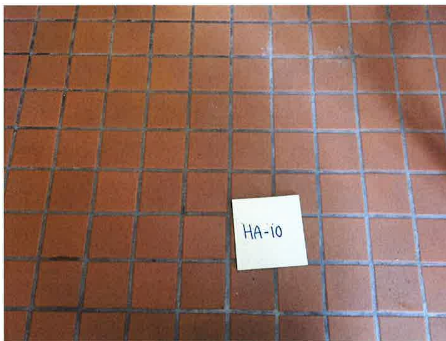
HA-10 Assumed asbestos-containing ceramic floor tile bedding compound and grout
