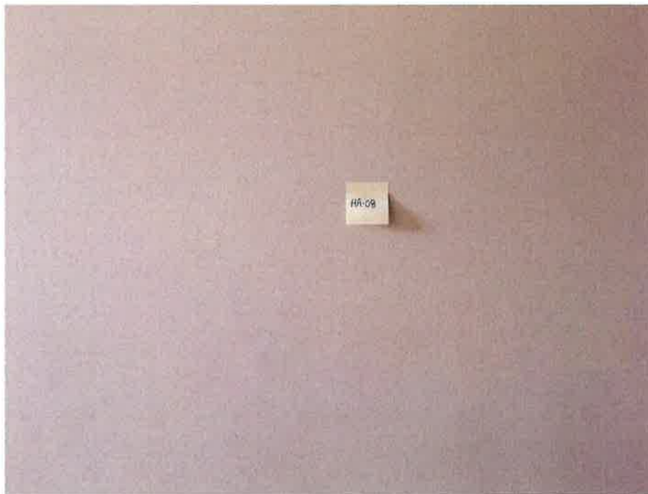
HA-08 Non-asbestos containing drywall
