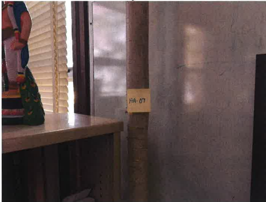
HA-07 Non-asbestos containing domestic water pipe straight insulation
