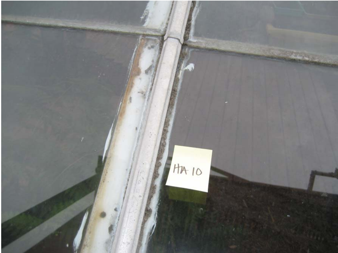
HA #10 – Asbestos containing gray and white exterior glazing compound, 1911 house
