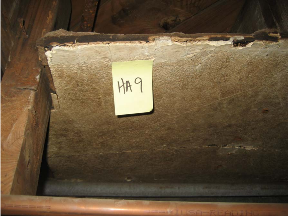
HA #9 – Asbestos containing 2'x 3' ceiling panel
