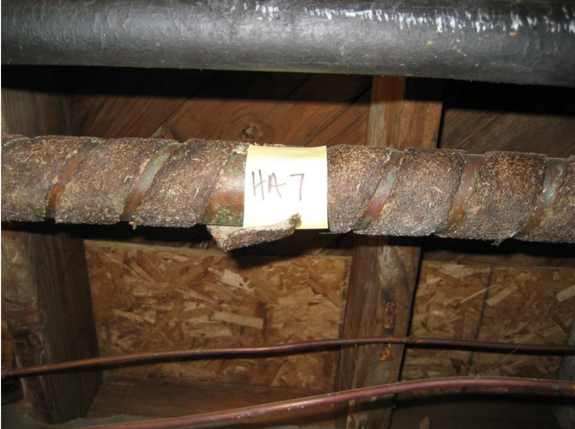
HA #7 – Asbestos containing black and brown pipe wrap
