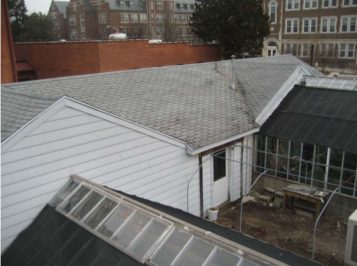
HA #11 – Asbestos containing Gray shingles, flashing, and associated mastics
