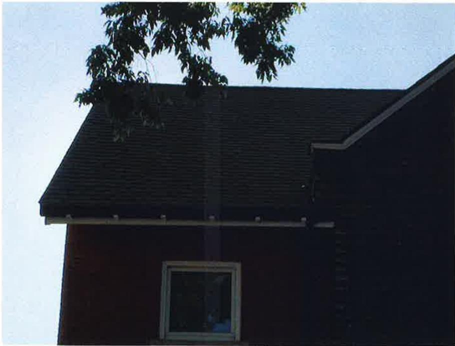
HA-27 Assumed asbestos-containing gray roof shingles and felts (tar paper)
