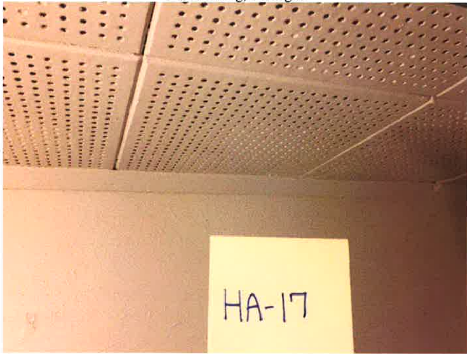
HA-17 Non-asbestos containing white 12" x 12" glued-on ceiling tile with uniform holes and HA-18 Assumed asbestos-containing gluepods
