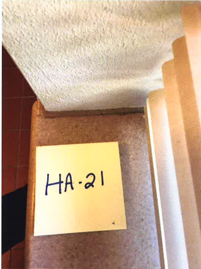
HA-21 Non-asbestos containing interior light brown window sill caulk
