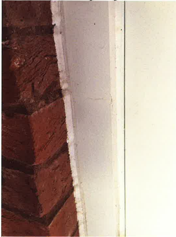
HA-28 Non-asbestos containing exterior white door caulk
