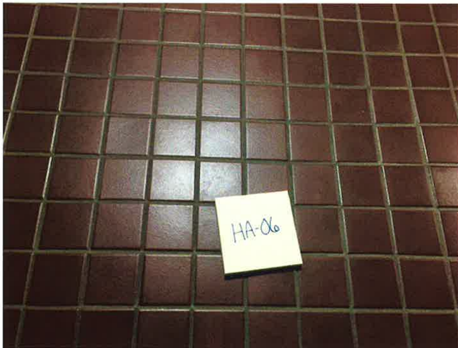
HA-06 Assumed asbestos-containing ceramic floor tile bedding compound and grout
