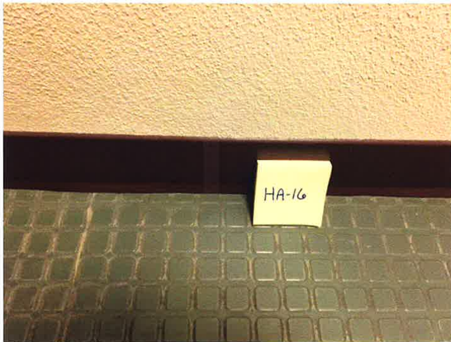
HA-16 Non-asbestos containing 4" maroon cove molding and associated mastic
