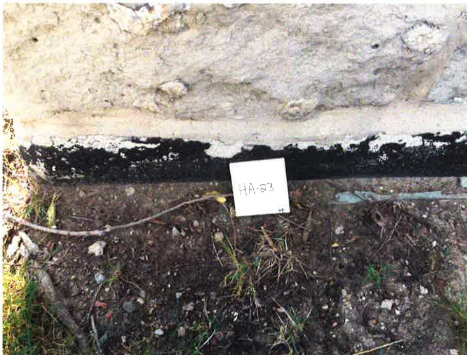
HA-23 Asbestos containing exterior black waterproofing
