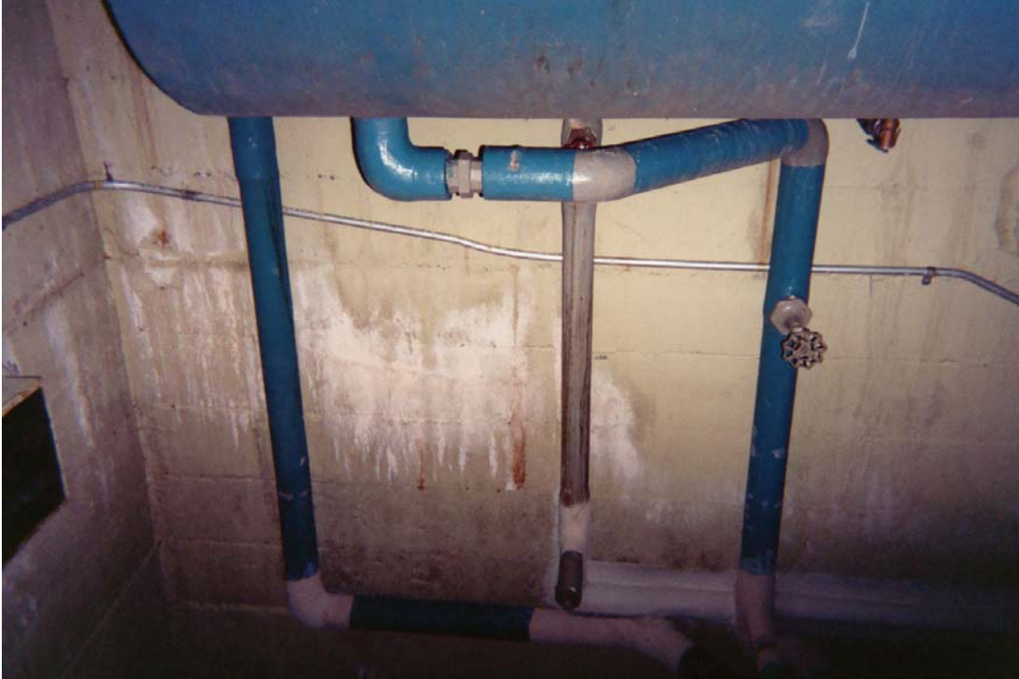
Photo 5 – Asbestos-containing domestic water supply and return pipe joint insulation
