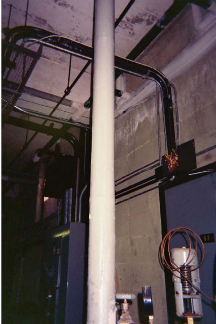
Photo 3 – Asbestos-containing steam/condensate supply and return pipe straight insulation
