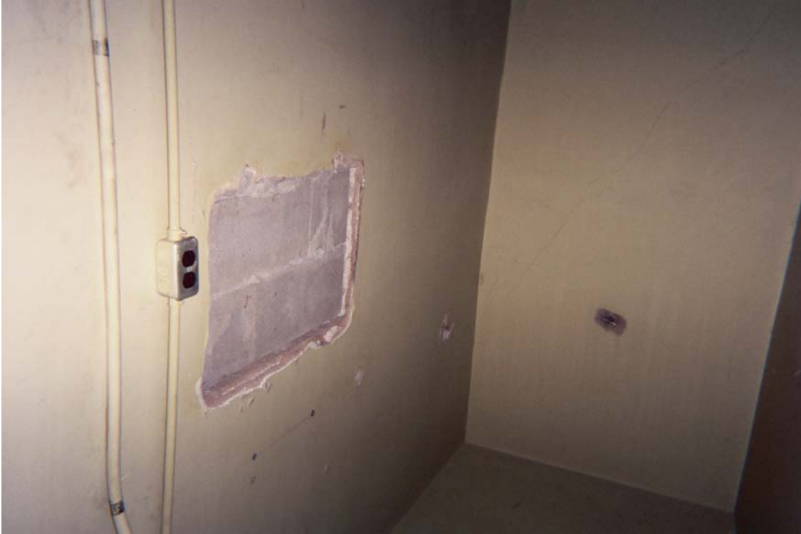
Photo 8 – Non asbestos-containing smooth plaster
