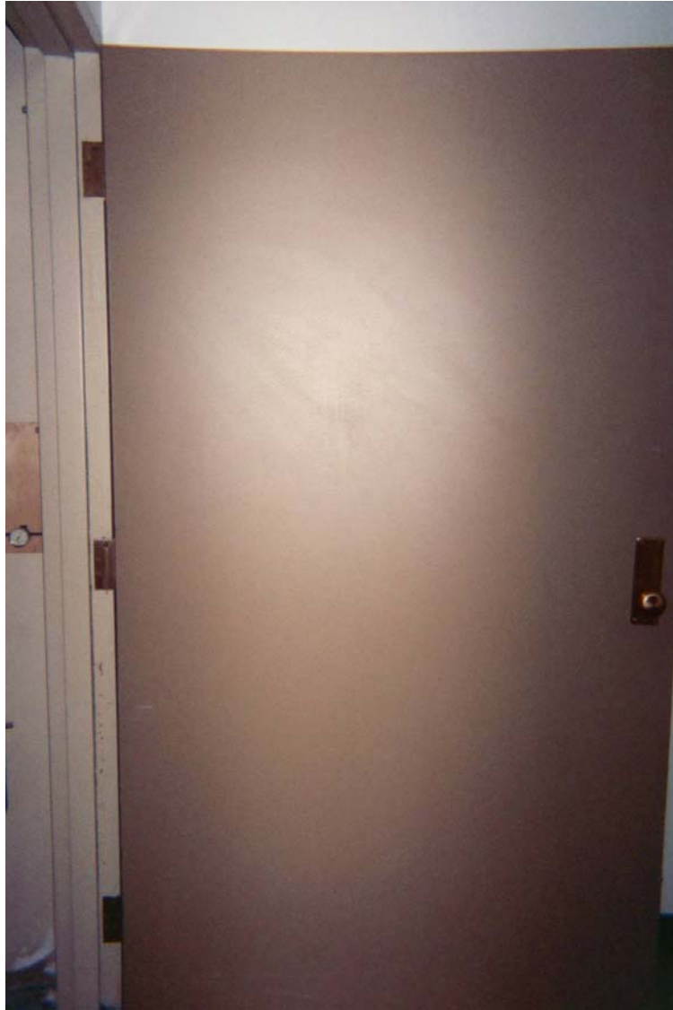
Photo 16 – Assumed asbestos-containing fire door and frame
