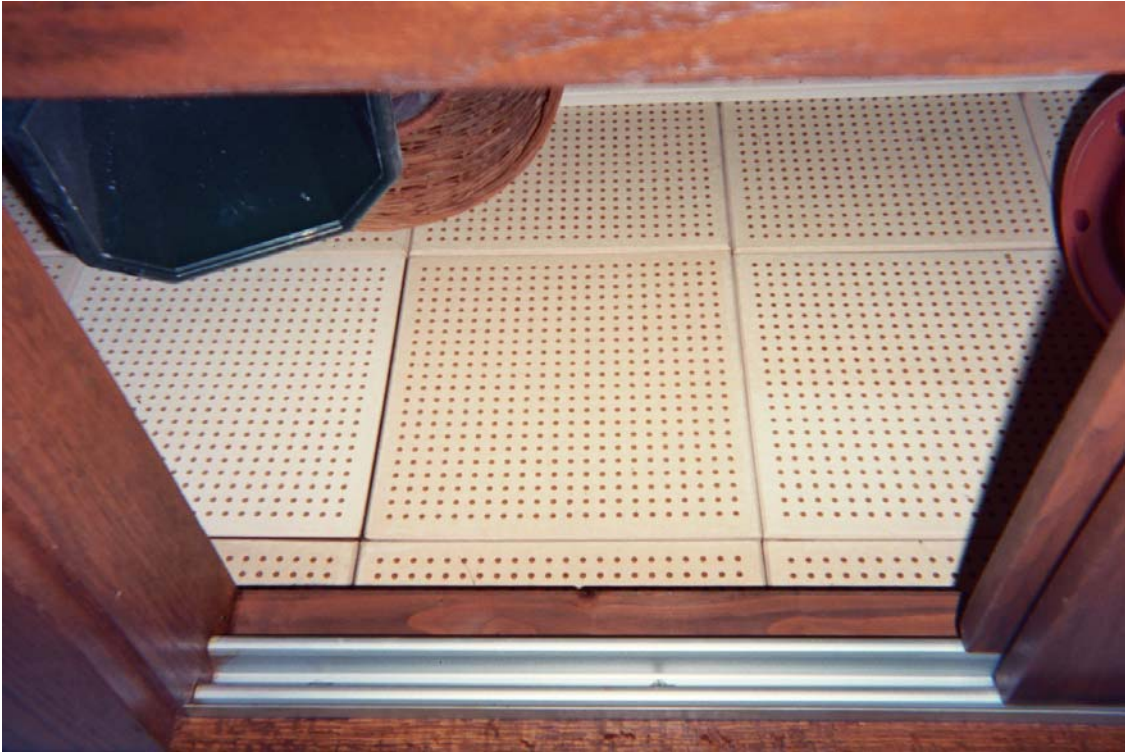
Photo 9 – Non asbestos-containing 12” x 12” white ceiling tile with uniform holes (glue pods are also non asbestos-containing)
